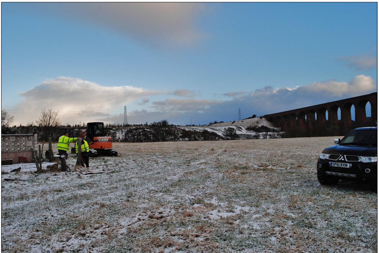
Plate 1 House site prior to stripping and the Nairn viaduct to right, facing N
