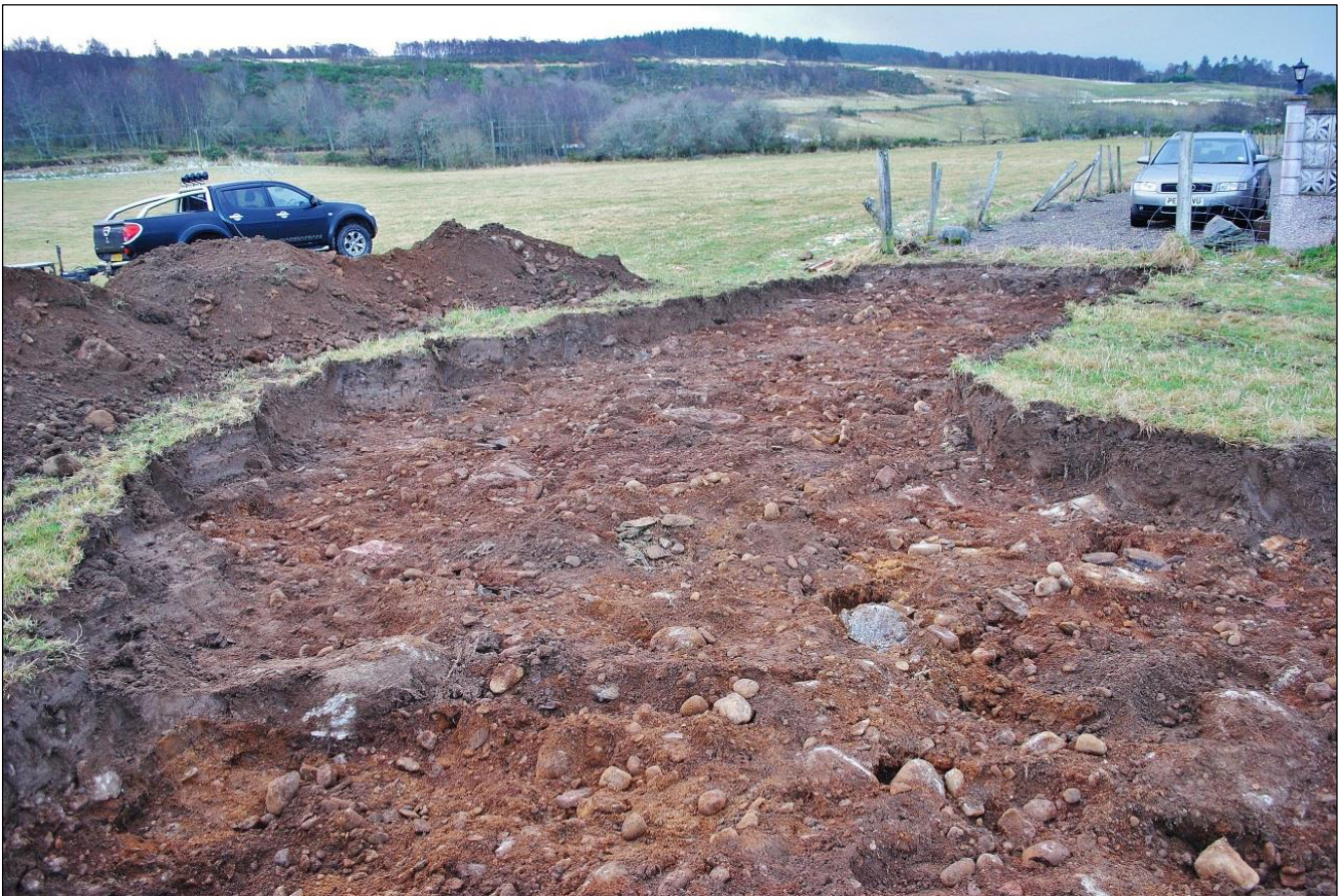
Plate 2 Driveway to the new house site after topsoil stripping, showing the stony and boulder-filled natural of the subsoil, facing S
