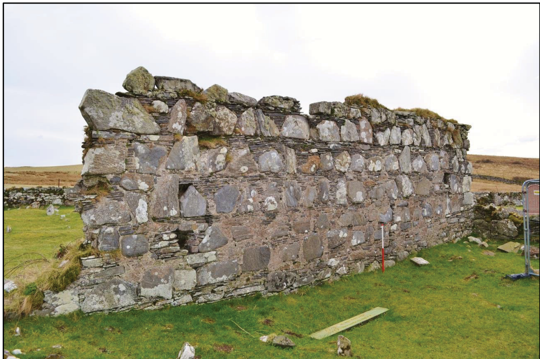
Plate 8: The interior face of the south wall, which is relatively intact (scale 1m)
