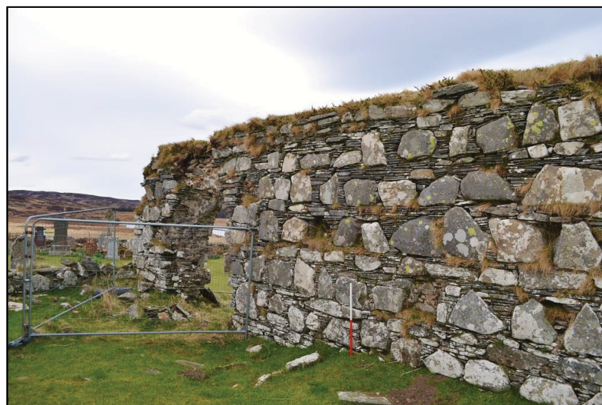
Plate 6: The internal face of the north wall; note the missing cladding stones (scale 1m)
