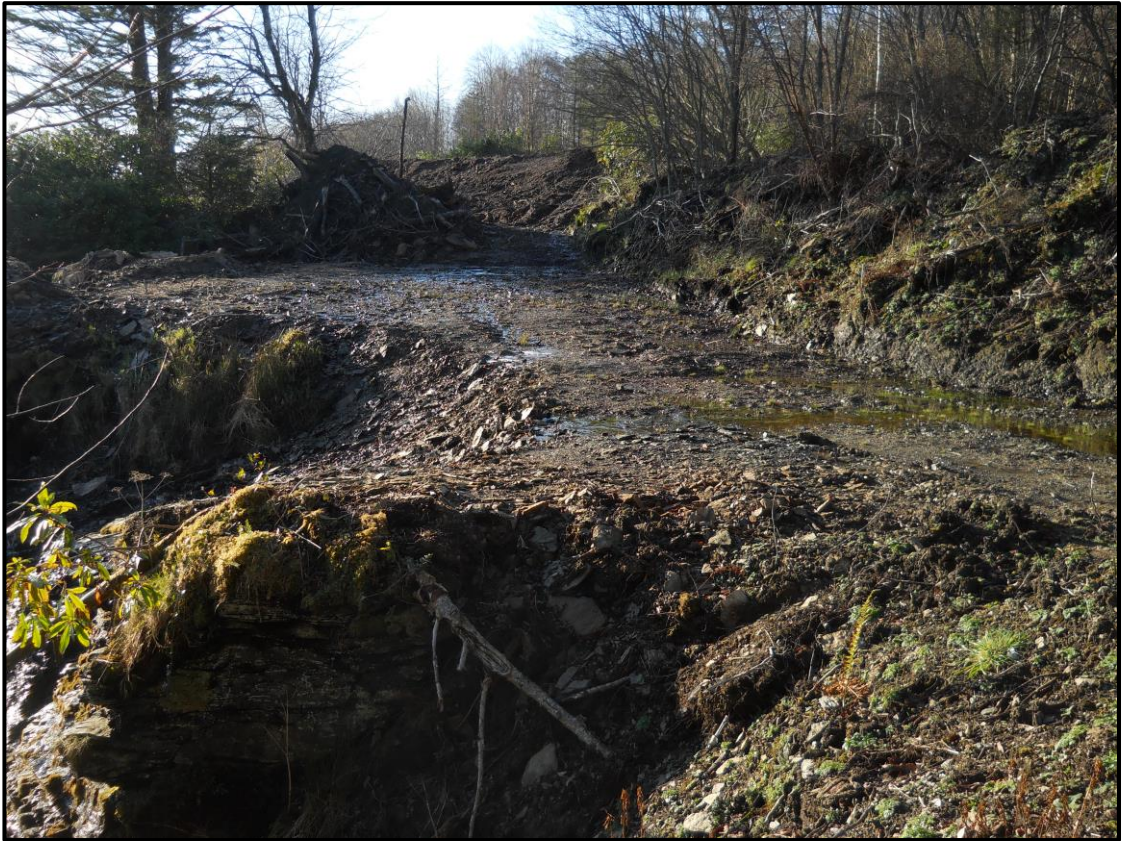
Plate 1: Looking over the narrow levelled platform of Plot 1 to the access cut leading up into Plot 2
