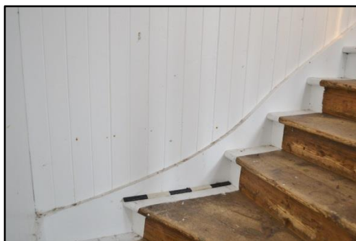
Plates 3, 4 and 5: (clockwise) these pictures show the staircase with curved panelling, the curved and re-curved skirting at the bottom of the stairs.
