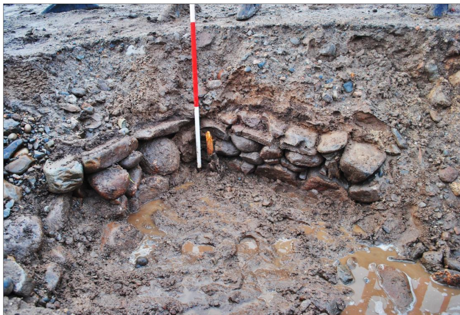
Plate 3 Feature 3: remains of a cobble-lined culvert / manhole over a drainage ditch; facing W
