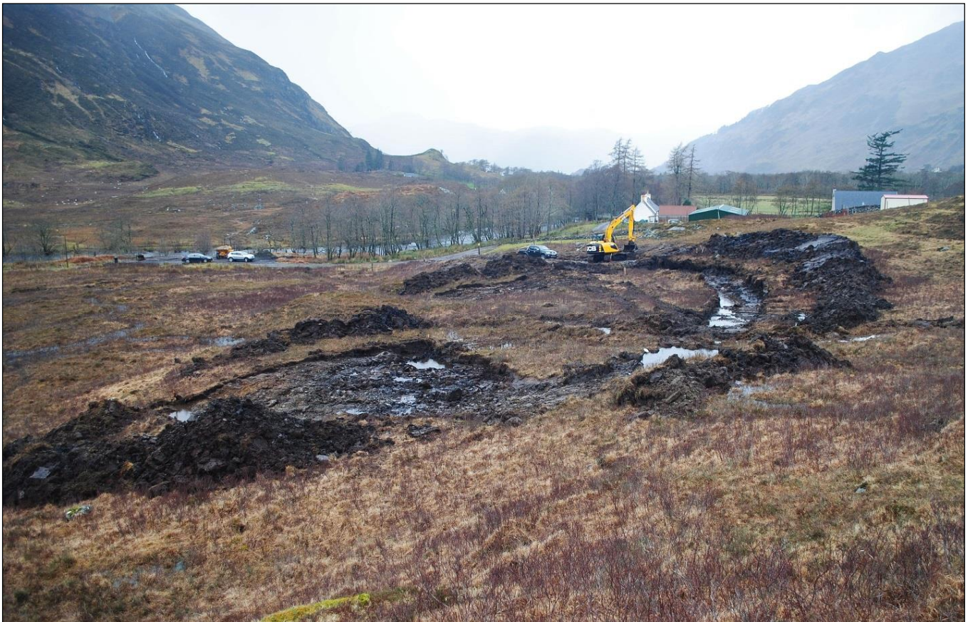
Plate 1 House sites and access track after site clearance, facing W with the River Croe in the background
