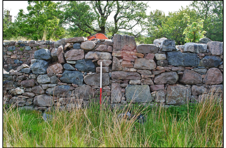
Plate 3: Visible join between north and south walls, west side of the building ruin
