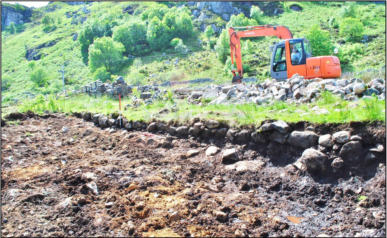
Plate 4: Looking southwest over the platform edge (Feature 3) during demolition of the ruin
