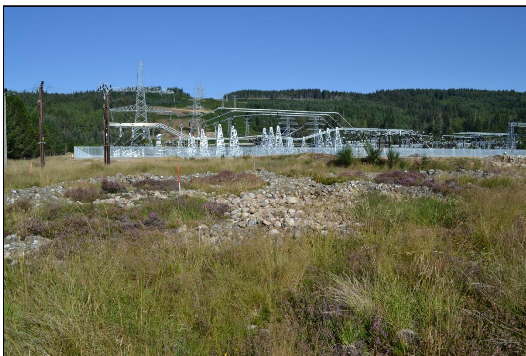
Plate 2: The large spread of stone looking N from the SW corner of the survey area
