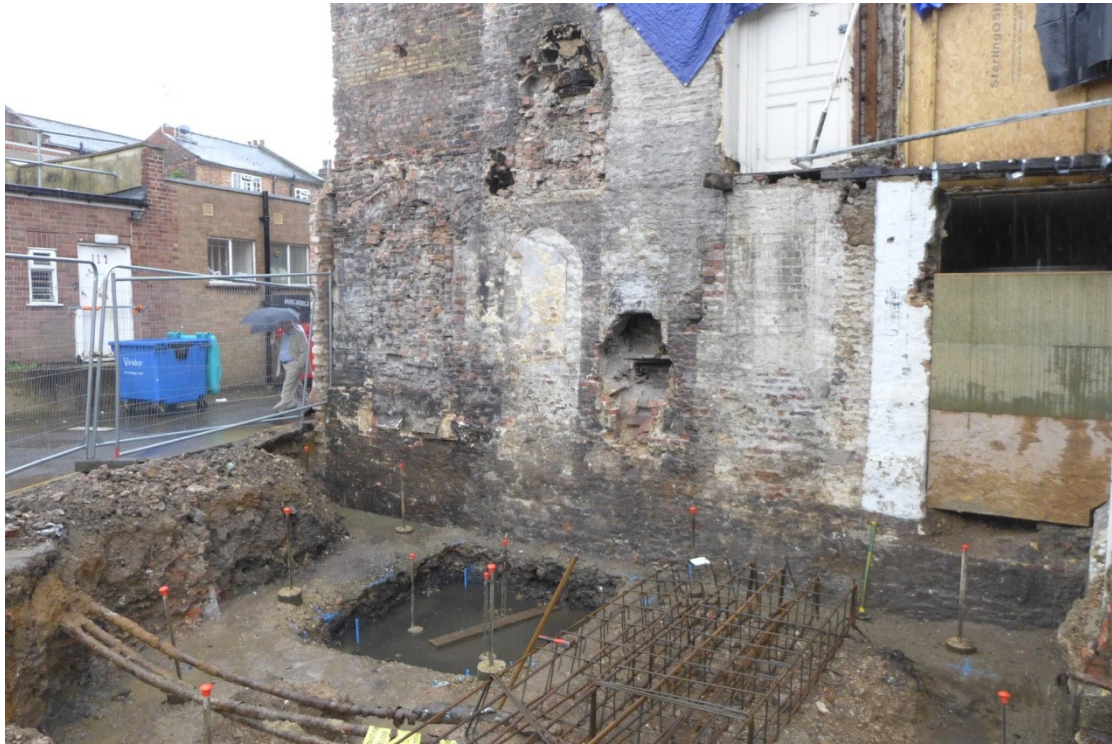
Plate 1: View of area north of the Old Gaol House after demolition of the store room and excavation for the foundations of the lift shaft. The area of the actual lift is represented by the smaller and squared deeper excavation in the central area.
