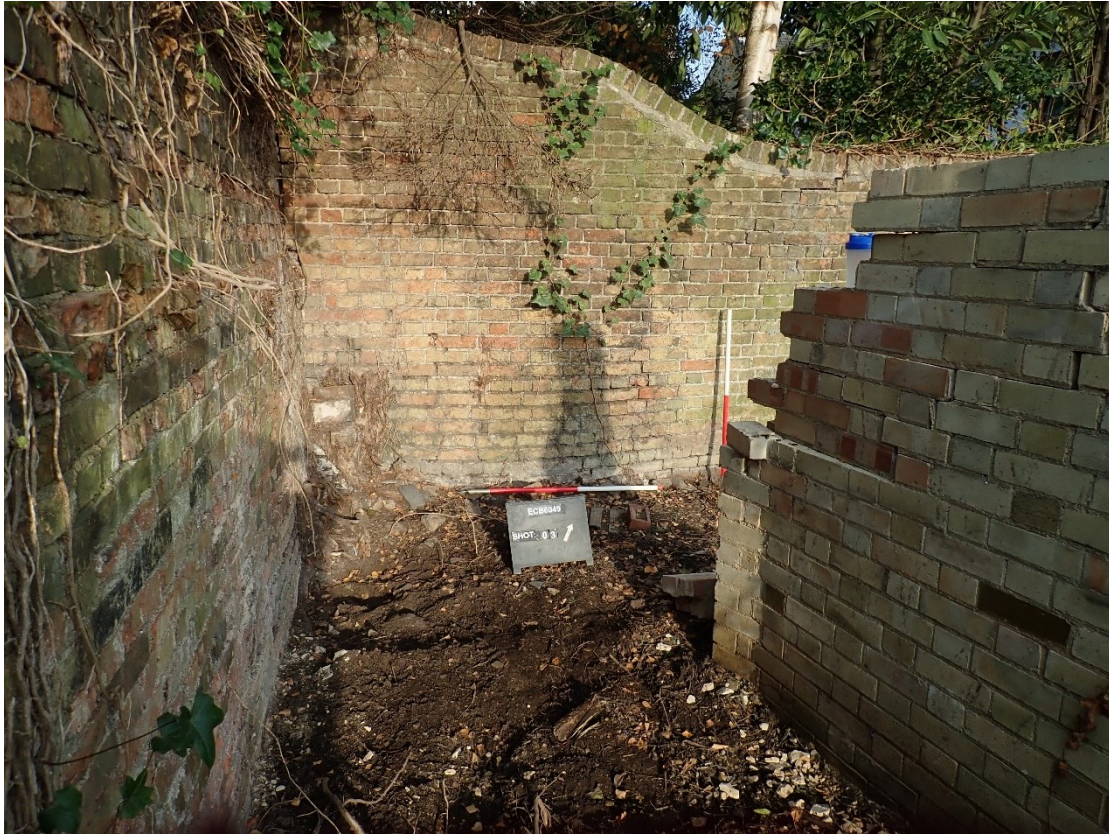
Plate 13: View of segment of north facing section of wall surrounding site (by north-west corner of wall), looking north, 2x1m scales
