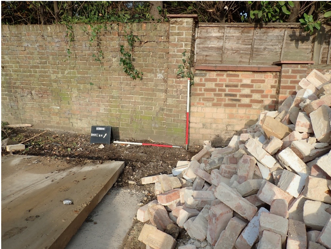
Plate 14: View of segment of north facing section of wall surrounding site, looking north-west, 2x1m scales
