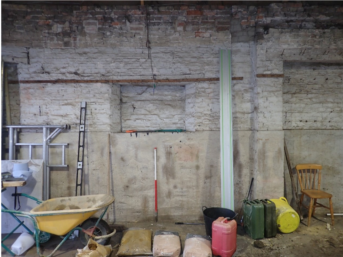
Plate 21: View of west inner wall rendering coat of workshop building, 1x1m scale
