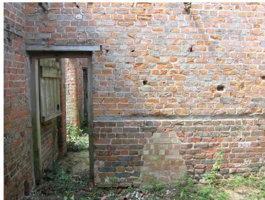
Plate 24: Building 2, Unit B – door to Unit A and repair in the internal wall
