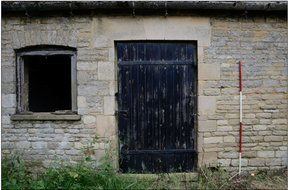
Plate 8: Door in the east wall of Building 5D, looking west-southwest (2m scale)
