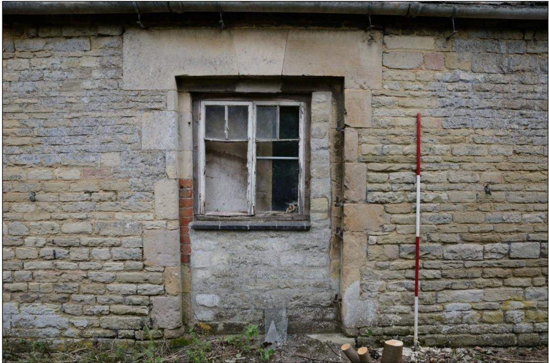
Plate 10: Former door in the east wall of Building 5C, looking west-southwest (2m scale)
