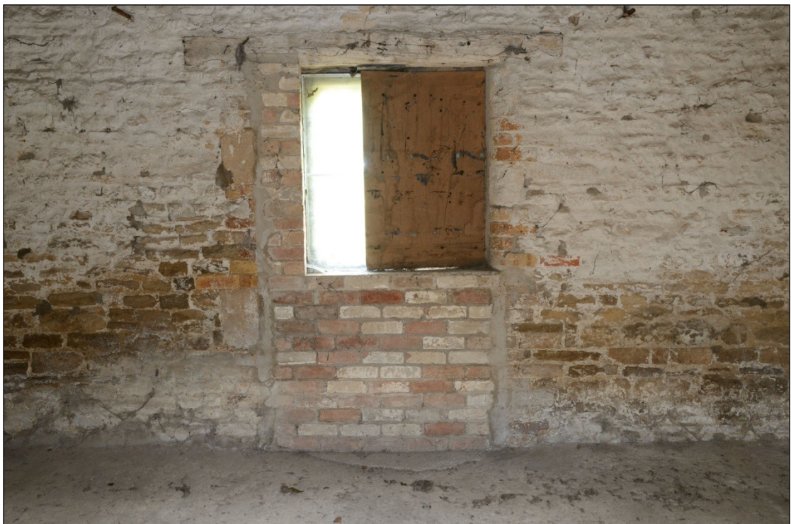
Plate 37: Blocked in doorway in the east wall of Building 5C, looking east-northeast
