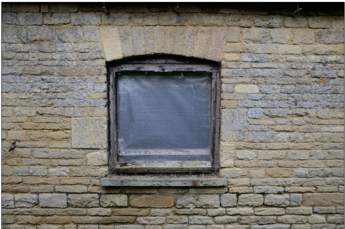
Plate 11: Window in the east wall, north of the door, of Building 5C, looking west-southwest
