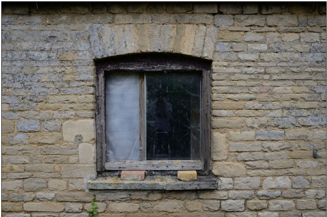
Plate 9: Window in the east wall, south of the door, of Building 5C, looking west-southwest
