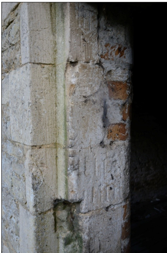
Plate 49: Graffiti on the south side of the door to Building 5D, looking southwest
