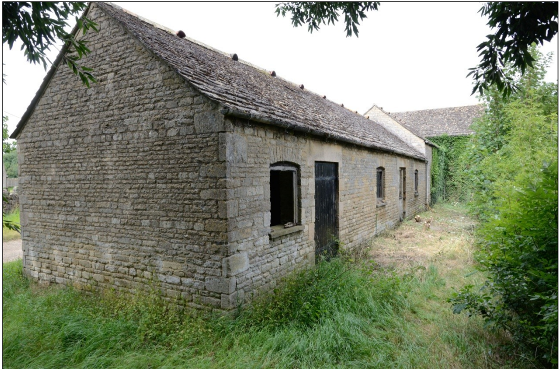
Plate 7: Building 5 (B, C and D), east and south facing elevations; looking northwest
