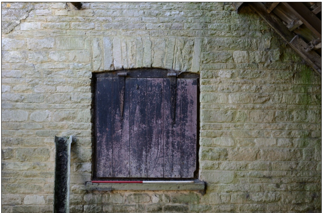
Plate 19: Window in the north facing elevation of Building 5A, looking south-southeast (1m scale)
