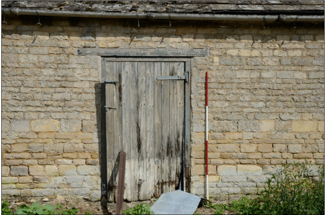
Plate 6: Door in the west wall of Building 5C, looking east-northeast (2m scale)
