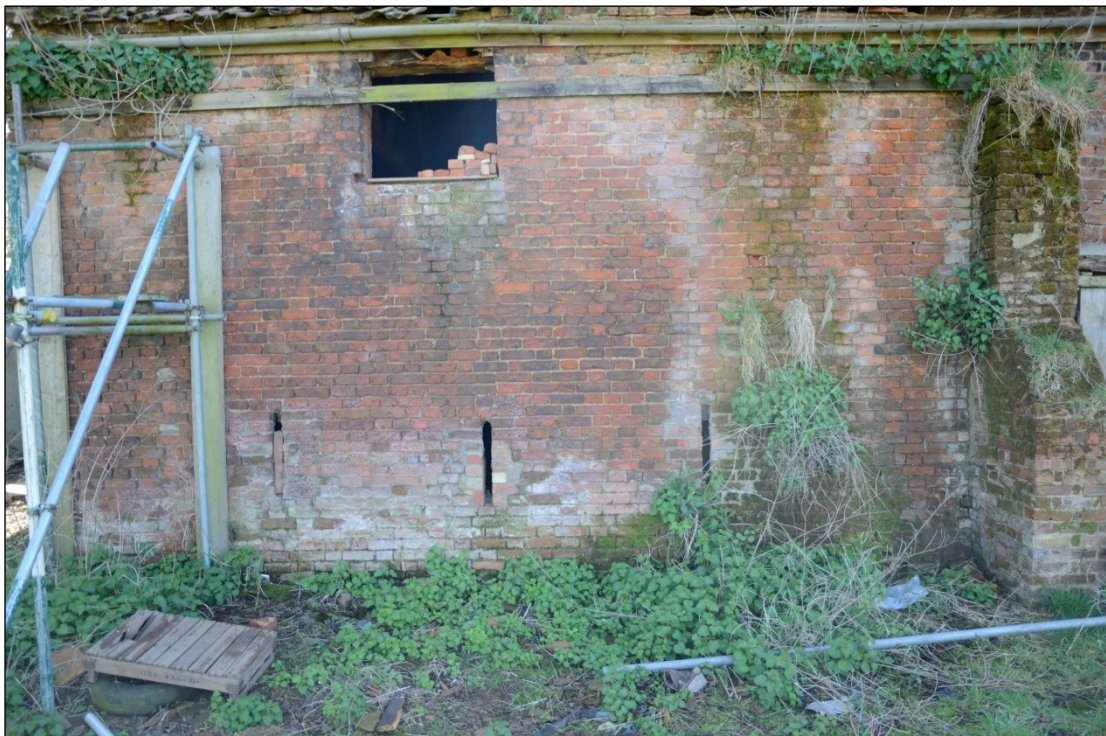
Plate 62: Ventilation slots in the north facing elevation (east end) of Barn 2, looking south
