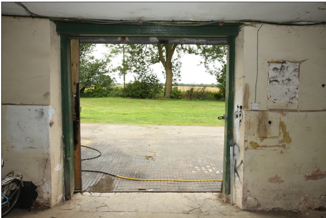
Plate 33: Interior of the door to unit at the eastern end of Building 1, looking north
