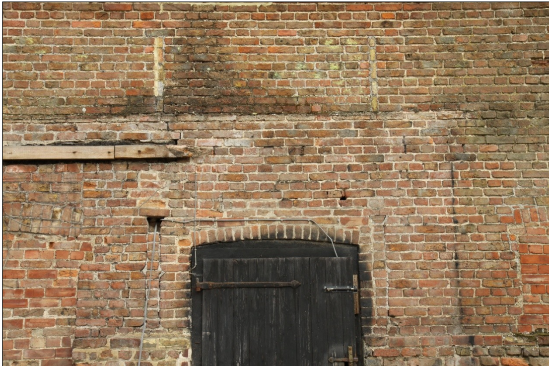
Plate 18: Ventilation slots around the existing door in the north elevation of Barn 1, looking south
