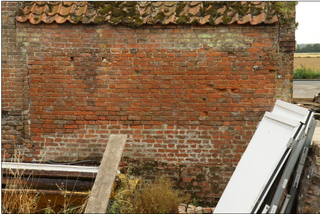
Plate 20: North facing elevation of the extension at the west end of Barn 1
