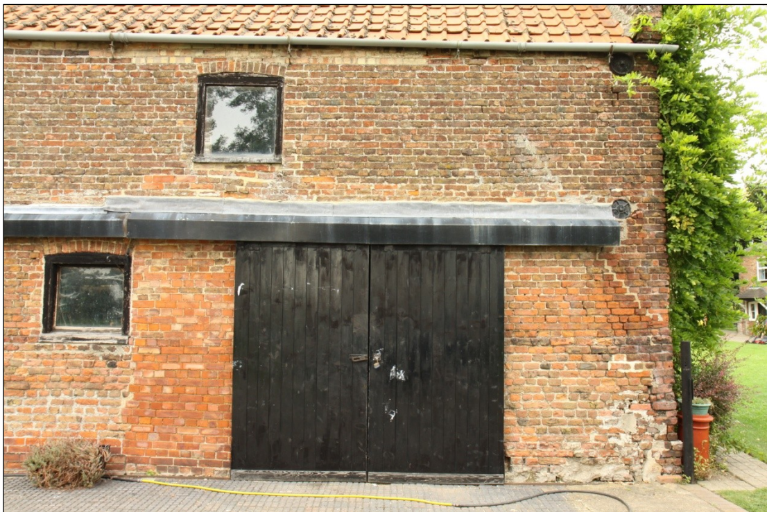
Plate 10: Door at the eastern end of the south facing elevation of Barn 1
