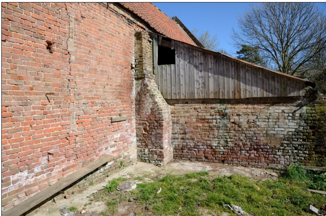
Plate 52: Junction of south facing elevation of Barn 2 and yard wall, looking northeast
