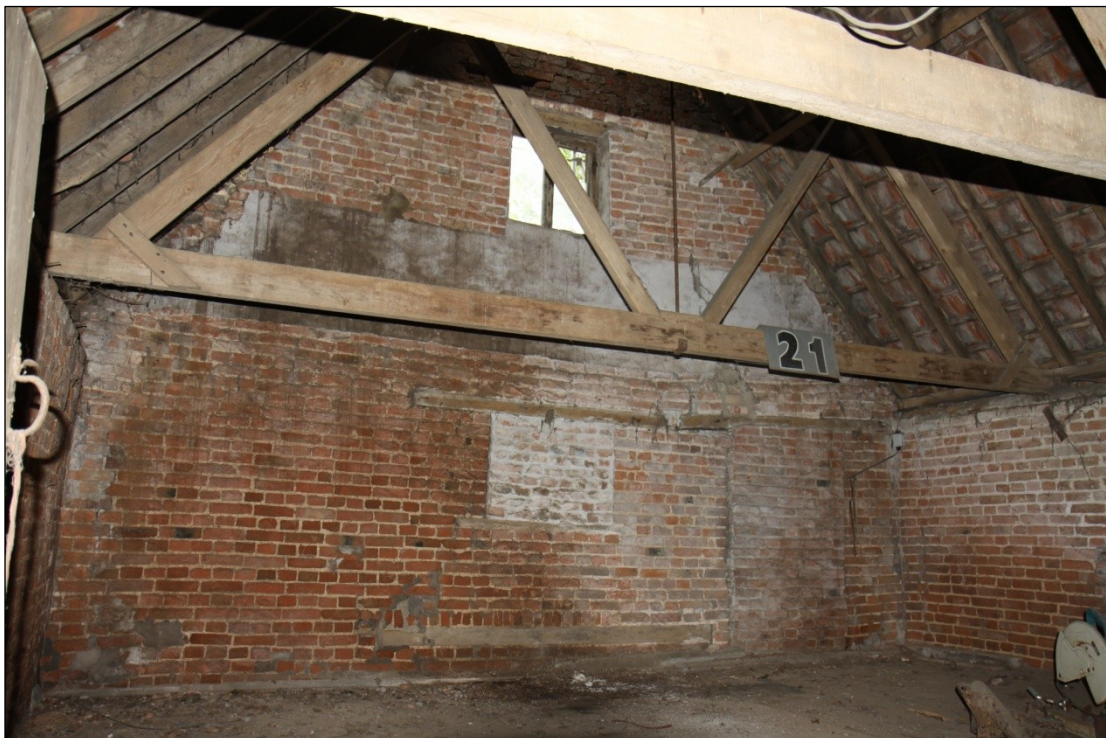
Plate 78: Interior of first floor unit (granary?) at the east end of Barn 2, looking southeast
