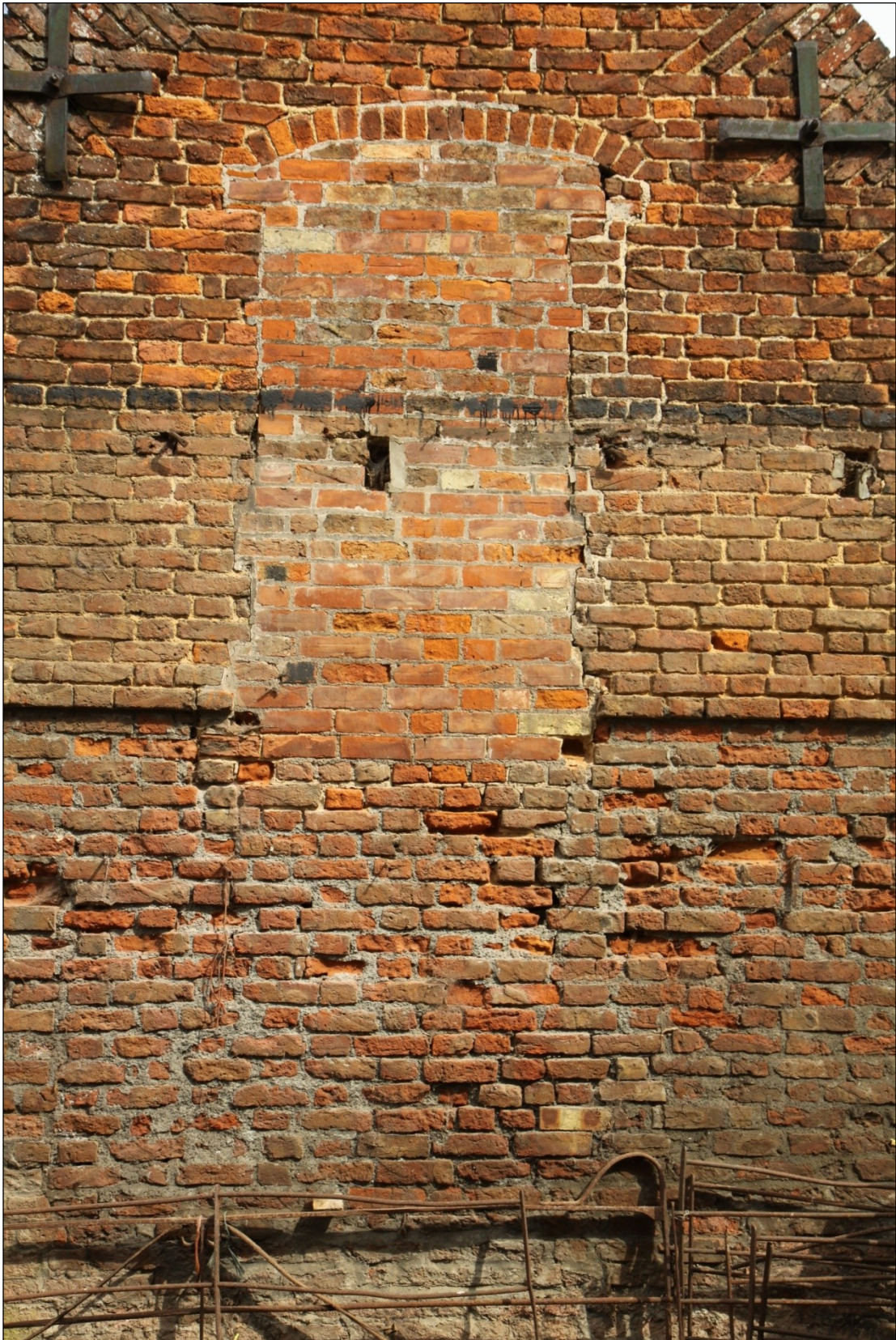
Plate 22: Blocked in doorway in the west facing elevation of the extension to Barn 1
