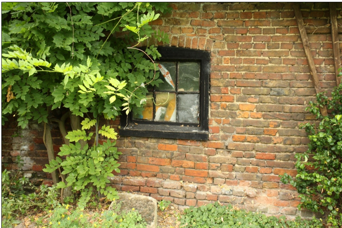
Plate 12: Ground floor window in the east facing elevation of Barn 1, looking west
