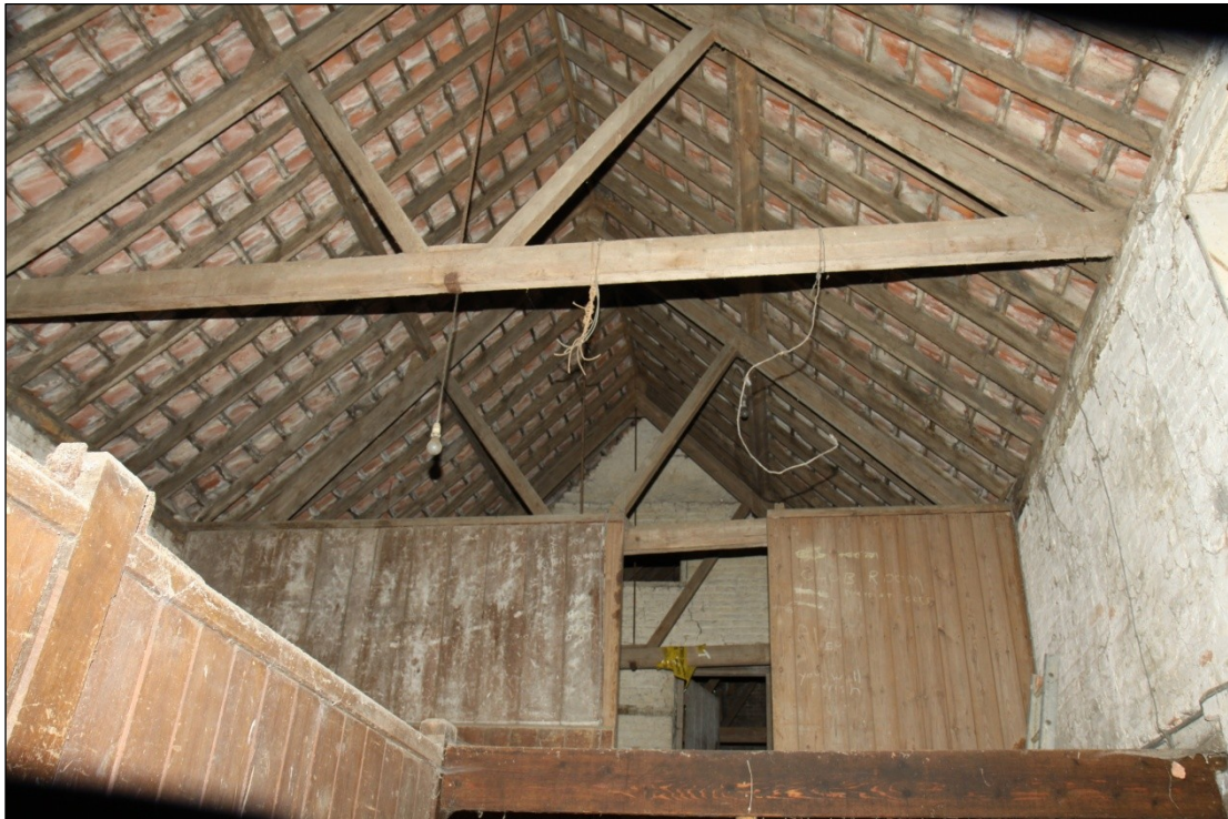
Plate 34: Hayloft and roof structure from the western end of Barn 1, looking east
