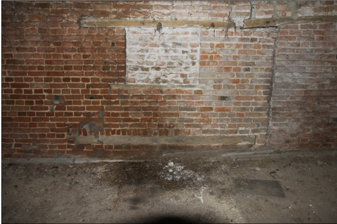
Plate 83: Timber lintel for ground floor opening at the east end of Barn 2, looking east
