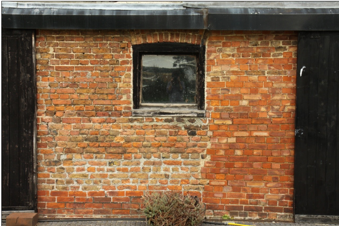
Plate 9: Ground floor window and modified doorway in the south facing elevation of Barn 1
