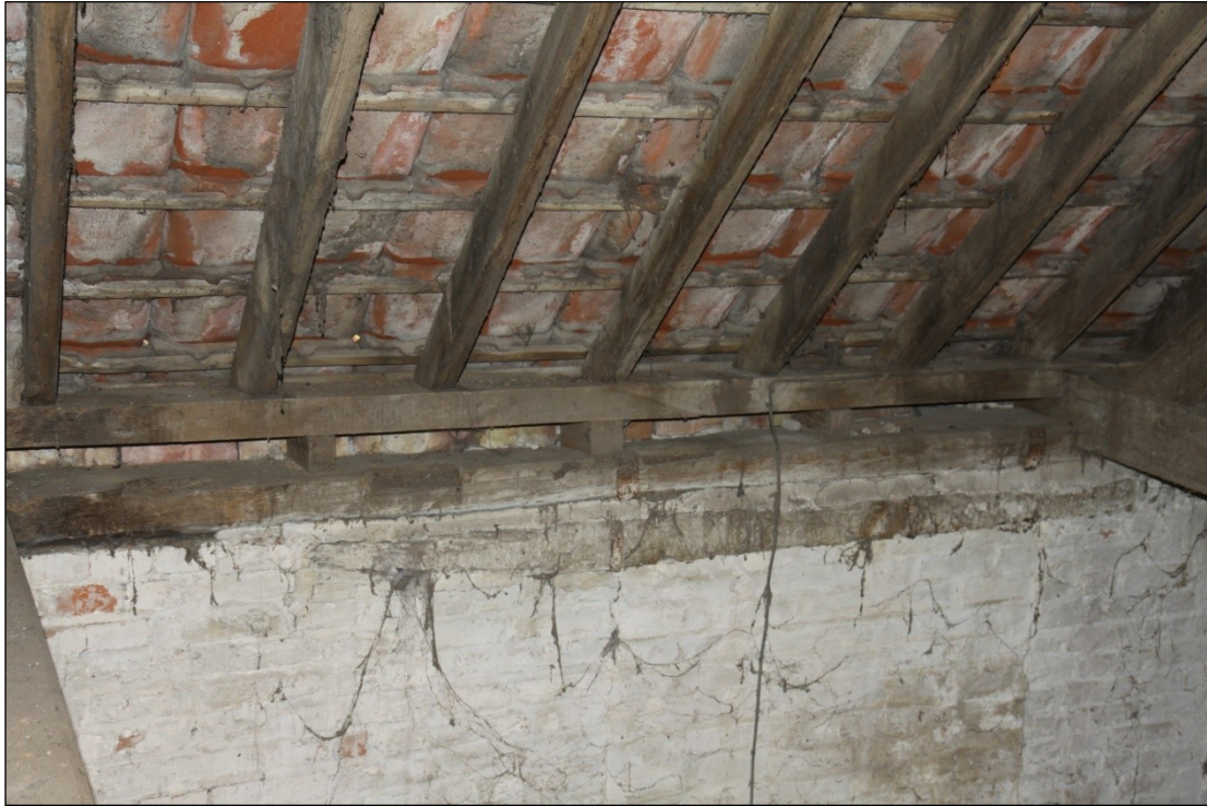
Plate 38: Bricked up opening (probable pitching door) in the south wall of Barn 1, looking southwest
