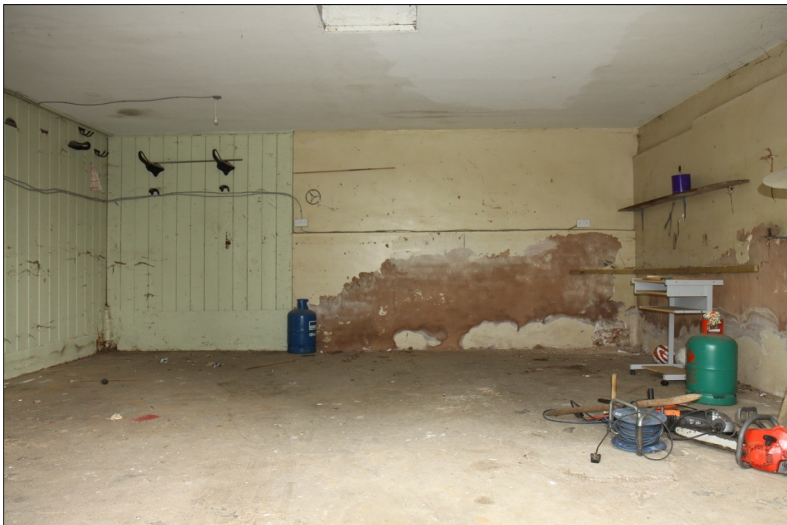
Plate 31: Unit including the former tack room at the eastern end of Barn 1, looking north
