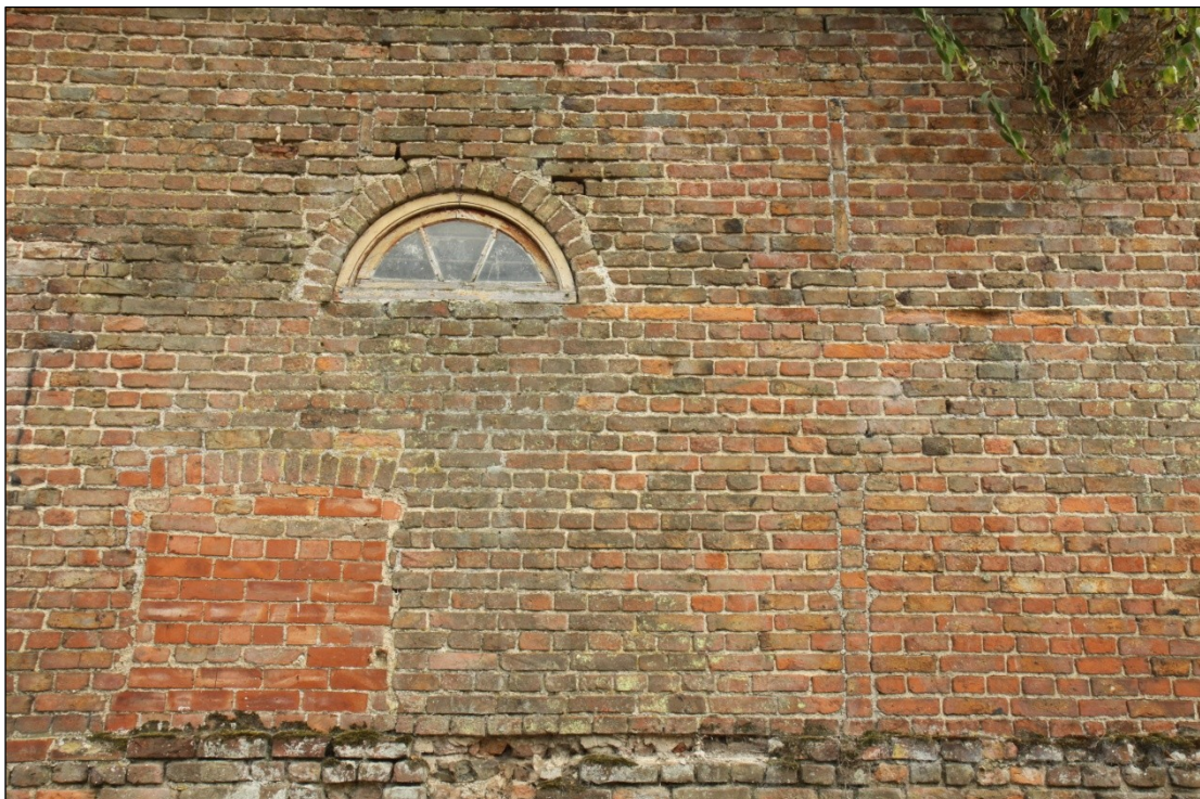
Plate 19: Ventilation slots, bricked up window, and fanlight in the north facing elevation of Barn 1
