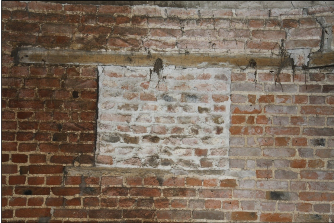
Plate 81: Bricked up vent or window in the east wall of Barn 2, looking east
