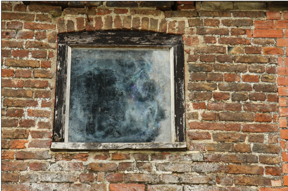
Plate 7: Second floor window located over ventilation slots in the south facing elevation of Barn 1
