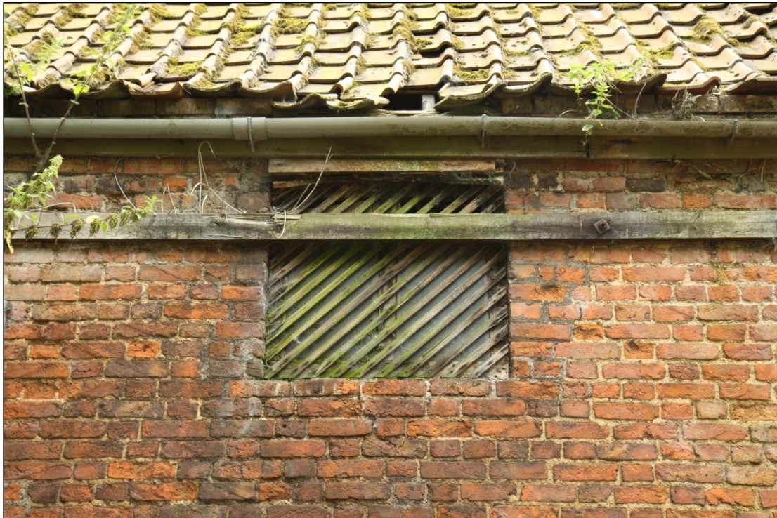
Plate 63: Vent or window to first floor in the north facing elevation of Barn 2, looking south
