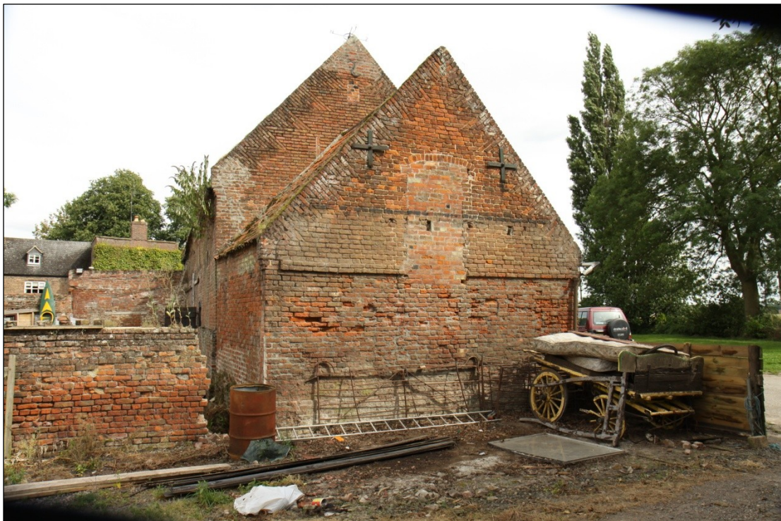
Plate 21: West facing elevation of the extension at the west end of Barn 1, looking ESE
