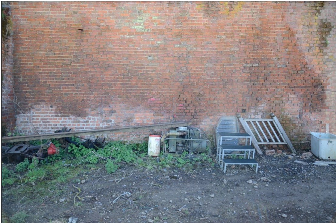
Plate 65: Ventilation slots in north facing elevation of Barn 2 (west side), looking south
