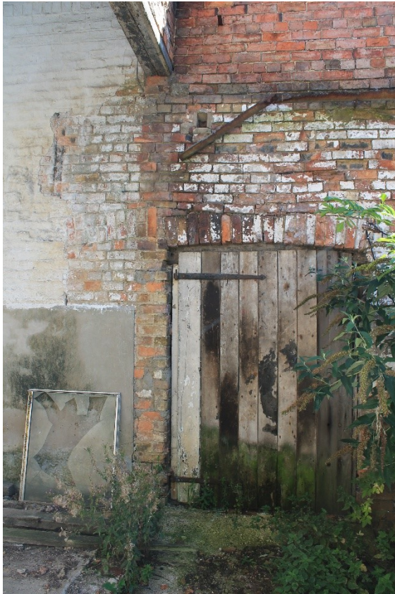
Plate 18 Detail of east wall of barn C, showing doorway, earlier blocked doorway to left, and position of southern wall of building B visible as vertical scar in whitewash, looking east.
