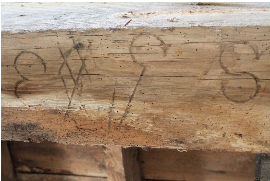
Plate 26 Possible carpenters marks or graffiti on underside of cart shed lintel (north bay), looking west/up.
