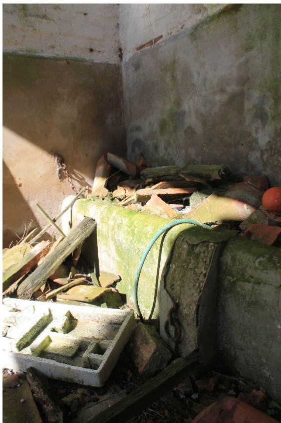
Plate 9 Interior of room B, detail showing rendered walls, concrete manger and iron tethering rings associated with use as cattle accommodation, looking northwest.
