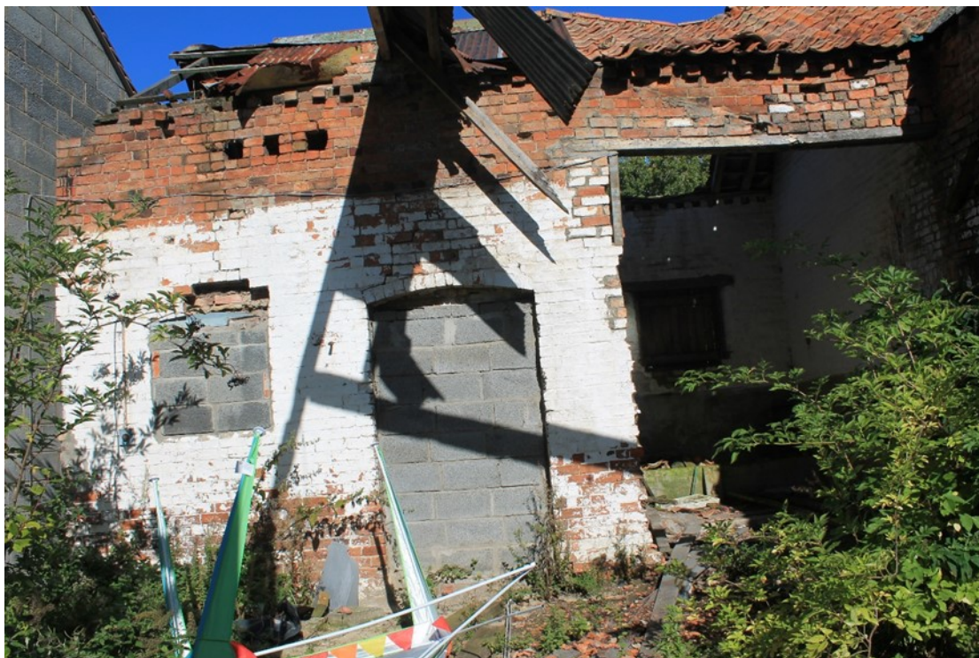
Plate 10 South external elevation of buildings A and B showing blocked openings of building A stable at left and three dove holes in brickwork at first floor level.
