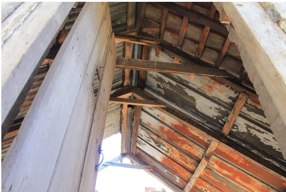
Plate 13 Interior of first floor dovecote of building A as viewed from doorway showing roof structure, looking west.
