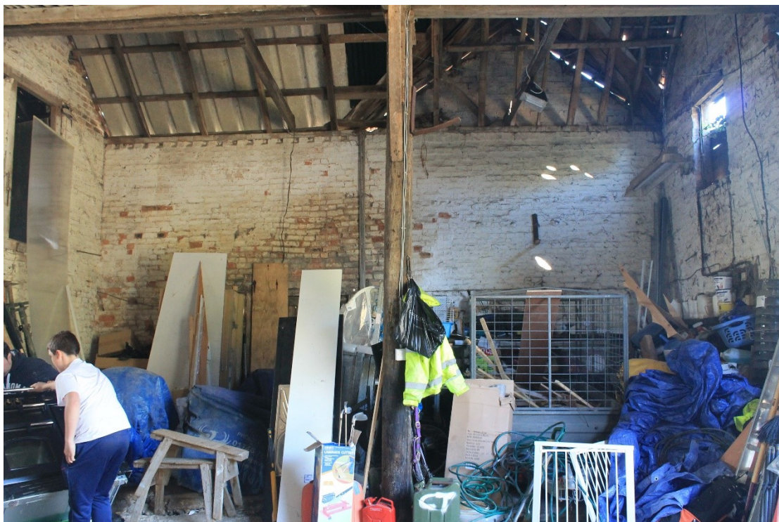
Plate 16 Internal view of west wall of barn C as seen from inside shelter shed D, looking west.
