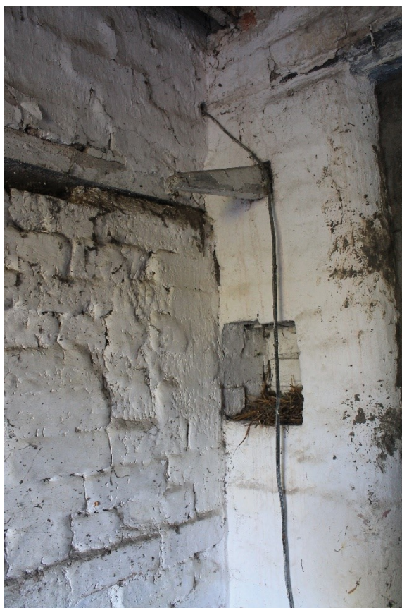
Plate 5 Interior of ground floor stable of building A showing tack hook and recess associated with use as stable, looking southeast.
