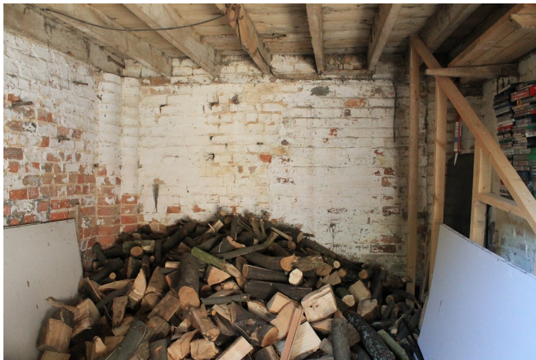
Plate 27 Interior of south bay of cart shed E, showing use of curved bricks at corners of building, possible tack hooks associated with later use as a stable at right and blocked doorway in west wall, looking west.
