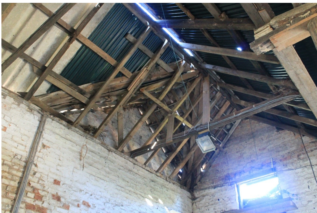
Plate 17 Interior of barn C (gable at right), detail of roof structure at junction with adjacent building B (gable at left), looking northwest.
