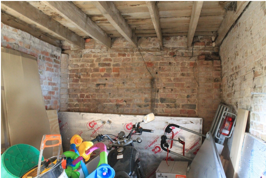
Plate 22 Interior of north bay of cart shed E, showing infilled brick wall at left and wooden joists and flooring of upper floor over, looking west.
