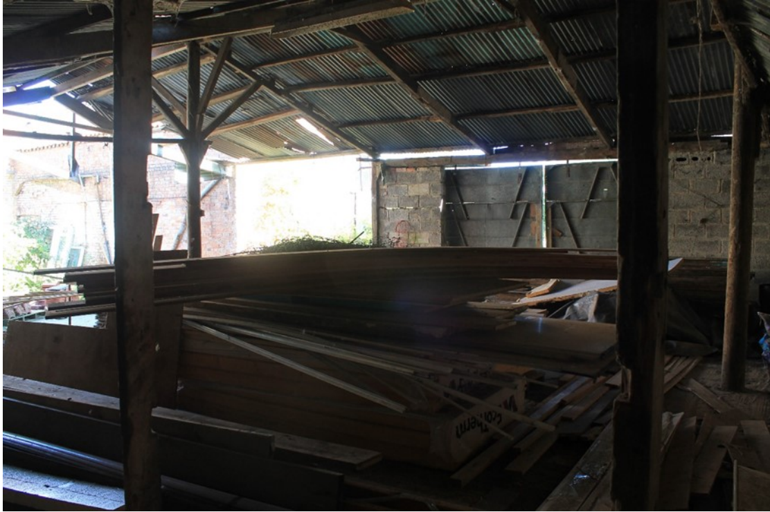
Plate 34 Interior of shelter shed I, showing wood, corrugated sheeting and breeze block construction, buildings E and C in background at left, looking northeast.
