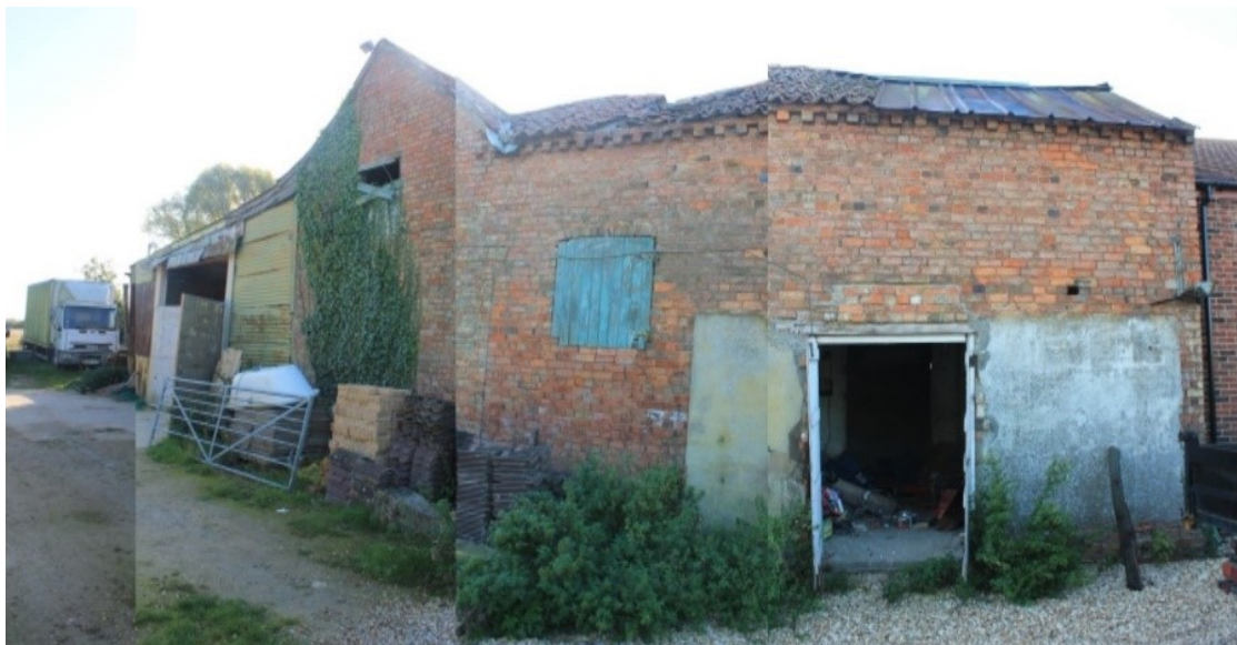
Plate 3 North elevation of surveyed outbuildings, dovecote and stable A at right, animal accommodation B at centre, Barn C at left and shelter shed D at far left, looking south and southeast.
