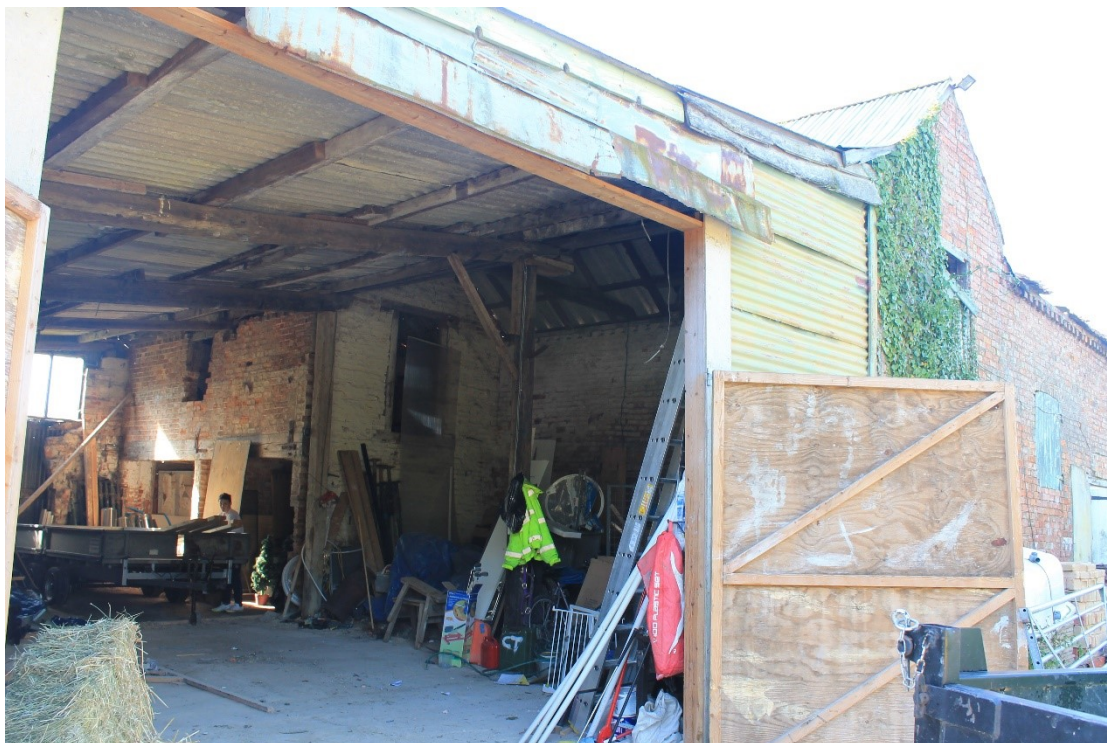
Plate 14 View of barn C, including external north gable end at right and south gable end now within shelter shed, looking southwest.
