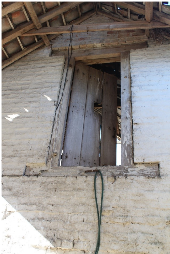
Plate 8 Doorway from room B leading to building A upper storey dovecote showing dove hole in plank door, looking west.
