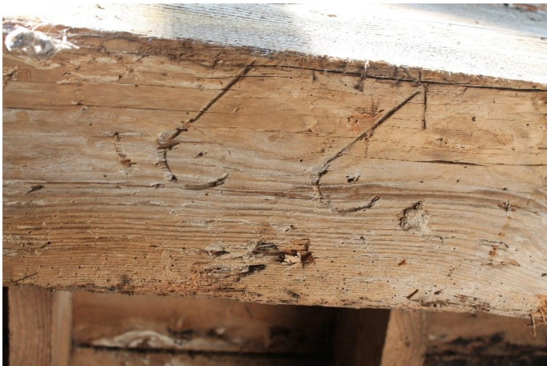
Plate 25 Possible carpenters marks or graffiti on underside of cart shed lintel (south bay), looking west/up.
