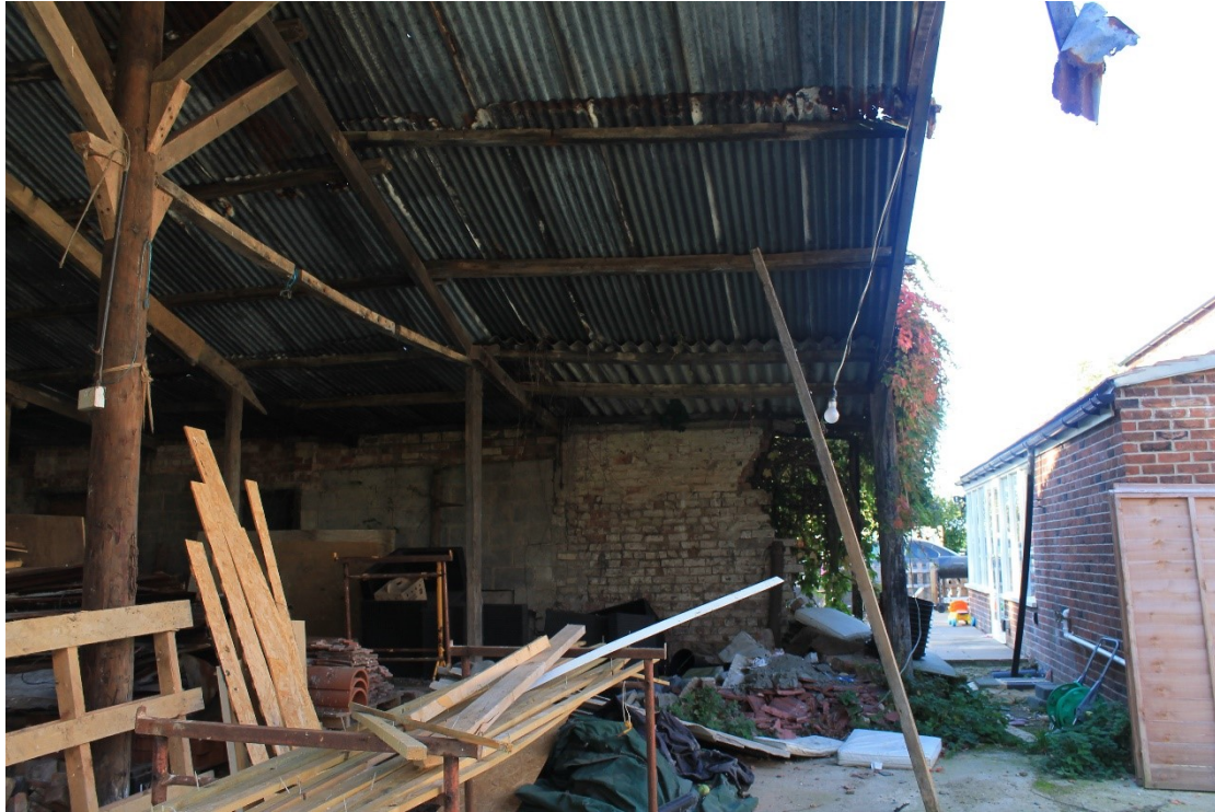
Plate 33, Interior of shelter shed I showing brickwork of western wall, conservatory and modern extension of farmhouse visible at right, looking west.
