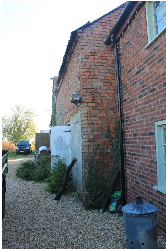
Plate 2 Northwest corner of outbuilding A showing slight coaching corner (modern farmhouse extension at right), looking east.
