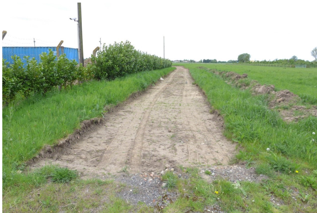
Plate 6: View of roadway leading to the site partially stripped of topsoil facing west
