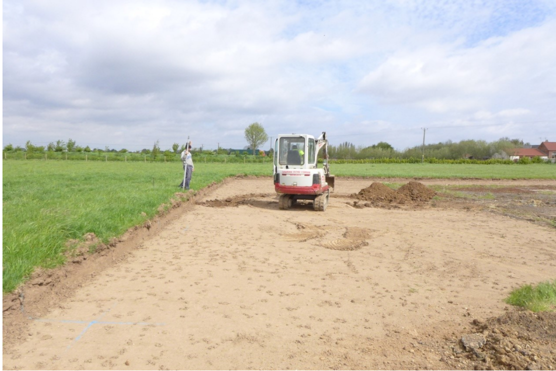
Plate 1: Work in progress. Excavation of the stanchion pits in the west area of the site
