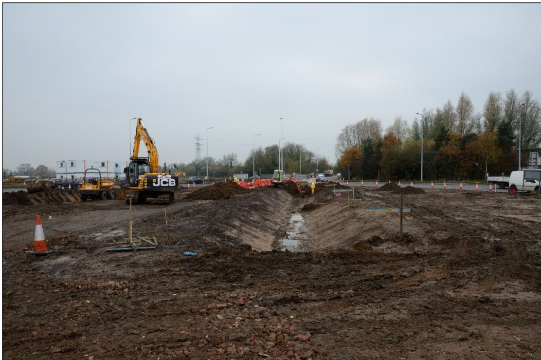
Plate 2: Work to upgrade headwalls in the existing ditch (Area C), looking west
