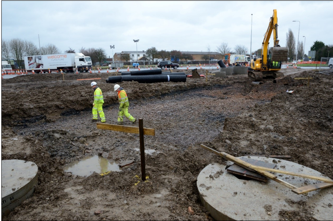
Plate 5: Work in progress to form the water storage feature (Area A), looking northeast
