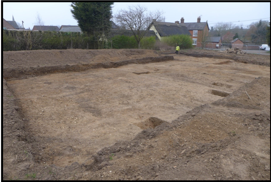
Plate 1: View of Area A under excavation facing southwest. The 18 th century thatched cottage known as 'Clay Walls' is visible in the background
