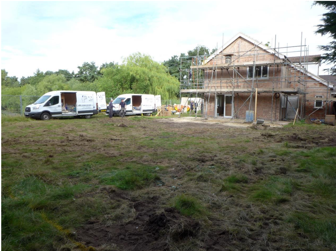
Plate 1: General view of site before topsoil stripping for car park, looking northwest
