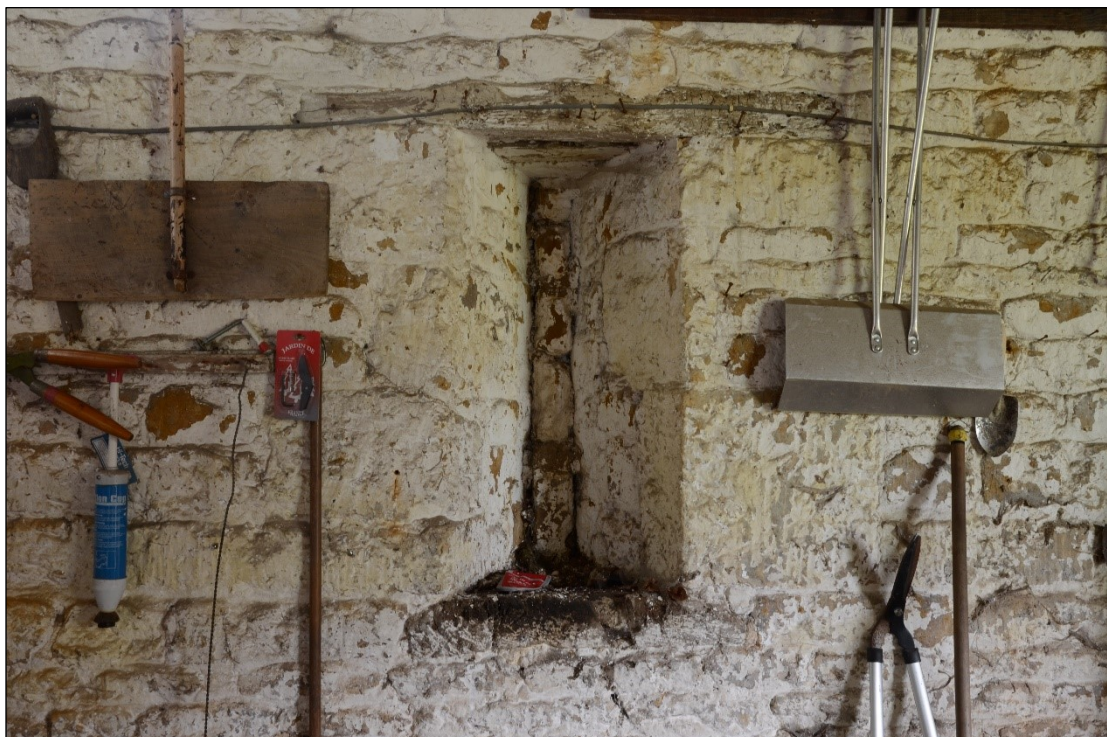
Plate 19: Blocked in vent in the southeast wall, northeast of the main door, looking southeast
