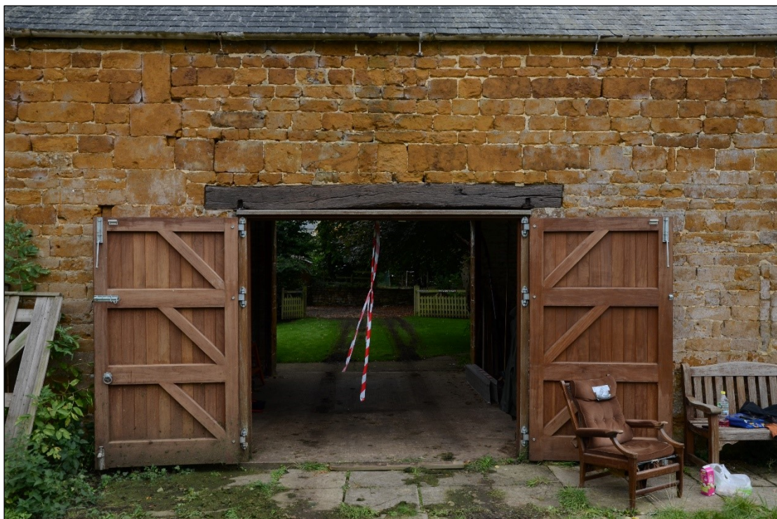
Plate 12: Door in the northwest wall, looking southeast (change in build, top left of door)
