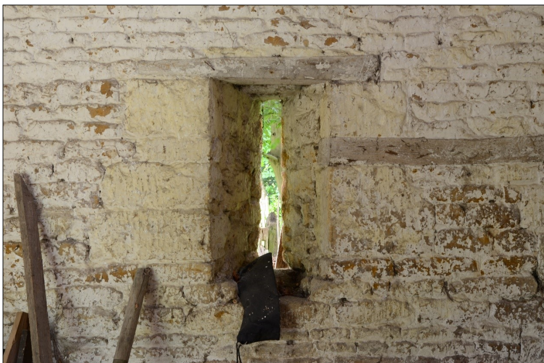
Plate 20: Vent in the southeast wall, southwest of the main door, looking southeast
