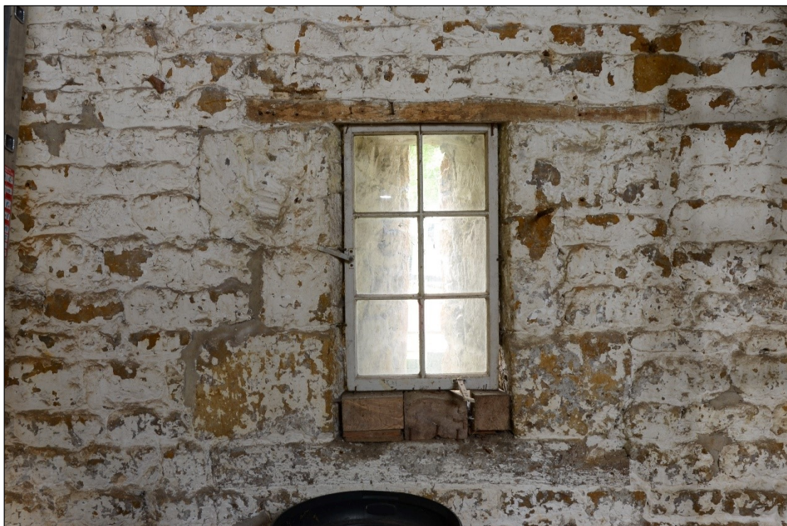
Plate 22: Window/ventilation slit in the northwest wall, northeast of the door, looking northwest
