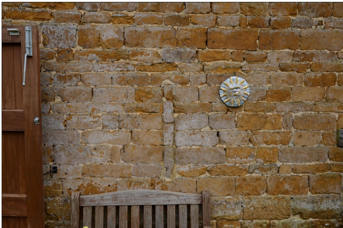
Plate 11: Blocked in vent in the northwest wall, southwest of the door, looking southeast
