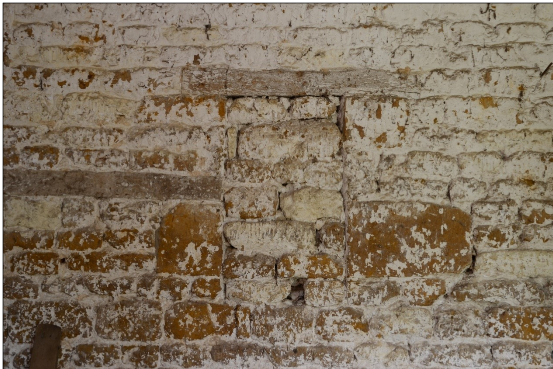
Plate 21: Blocked in vent in the northwest wall, southwest of the door, looking northwest
