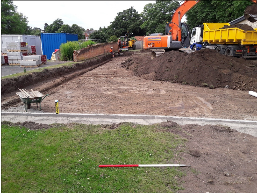
Plate 5: General view of stripped area on the southern side of the site, looking west; scale 1m
