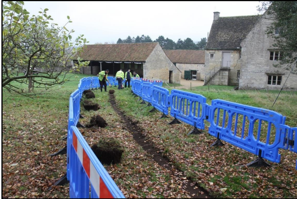
Plate 1: General view of turf removal at north end of cable trench, looking southwest towards Manor and outbuildings
