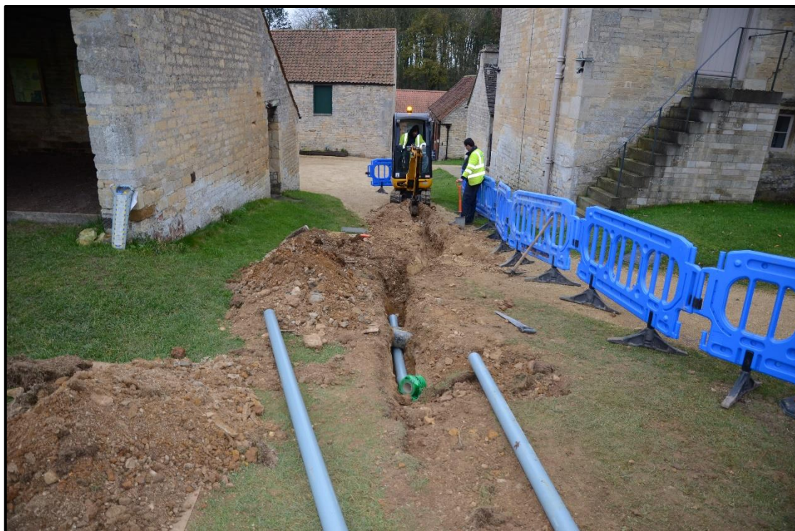
Plate 7: General view of trenching between manor house (to right) and farm buildings, looking south
