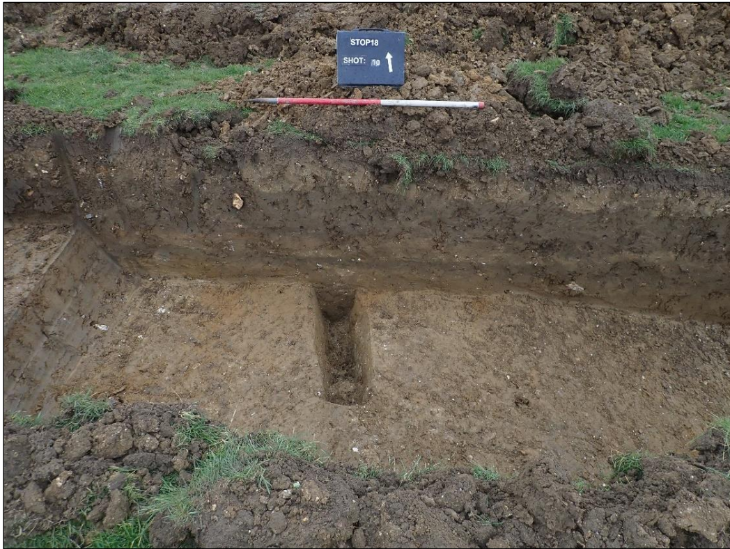
Plate 3: General view, looking northwest (NW end part excavated; leaving drain intact): 1m scale
