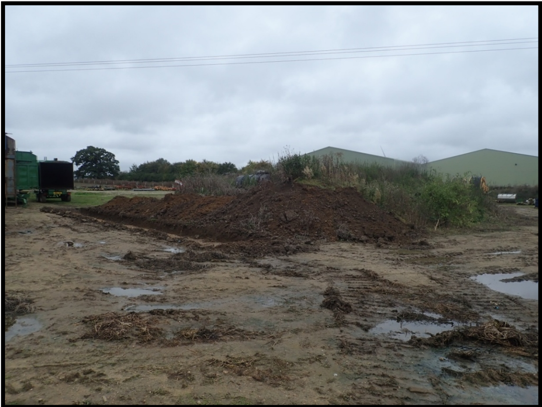
Plate 4: View of the southeast part of the development site looking over Trench 16 facing southwest
