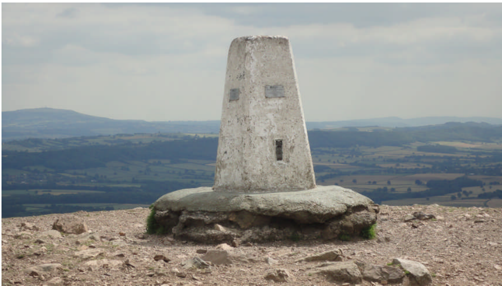
Photo 2: The triangulation point, showing the erosion at its base; looking southeast
