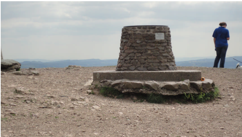
Photo 3: The toposcope, showing the erosion at its base; looking southwest
