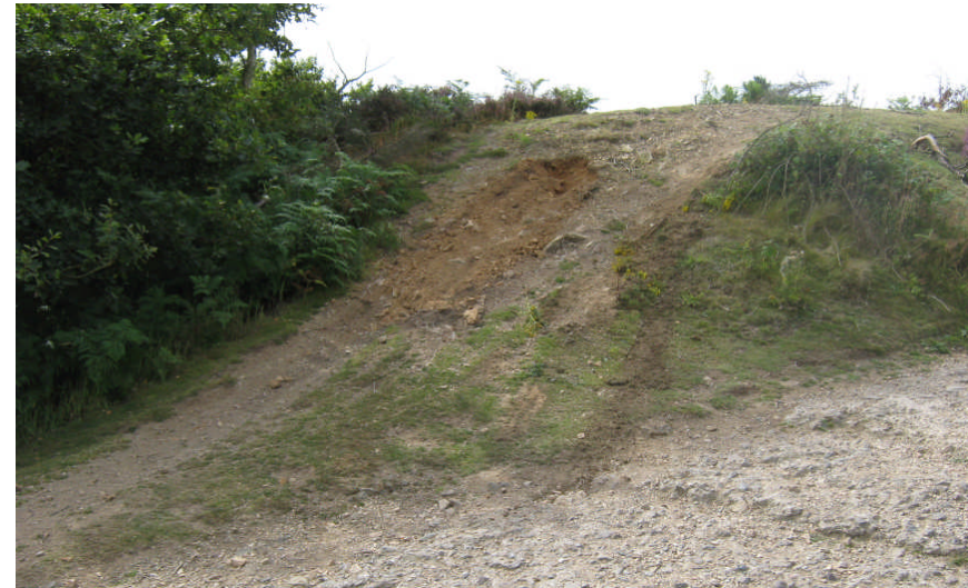
Photo 7: Recent damage to the Hell's Gate (outer northeast) entrance, probably caused by a 4x4 off-road vehicle
