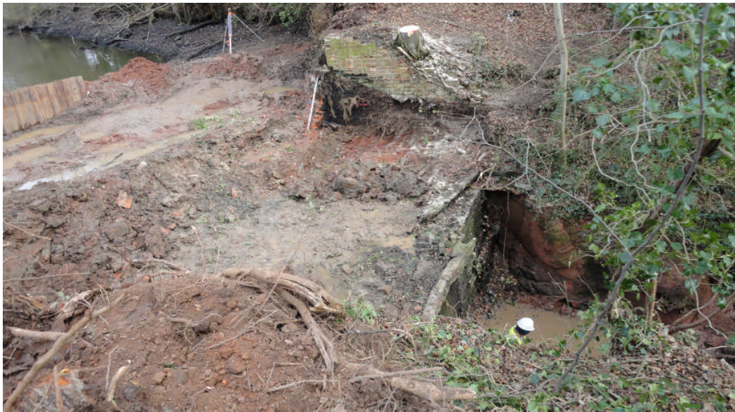
Photo 5: The weir and spillway during work to reduce the crest of the weir, looking NE
