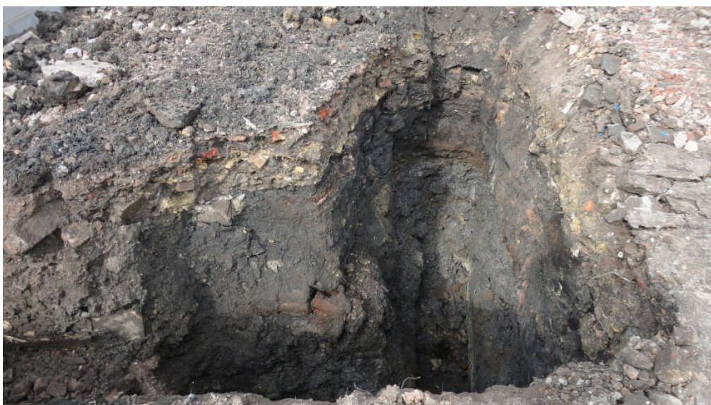
Photo 6: Deep industrial tip deposits in the central part of the development area
