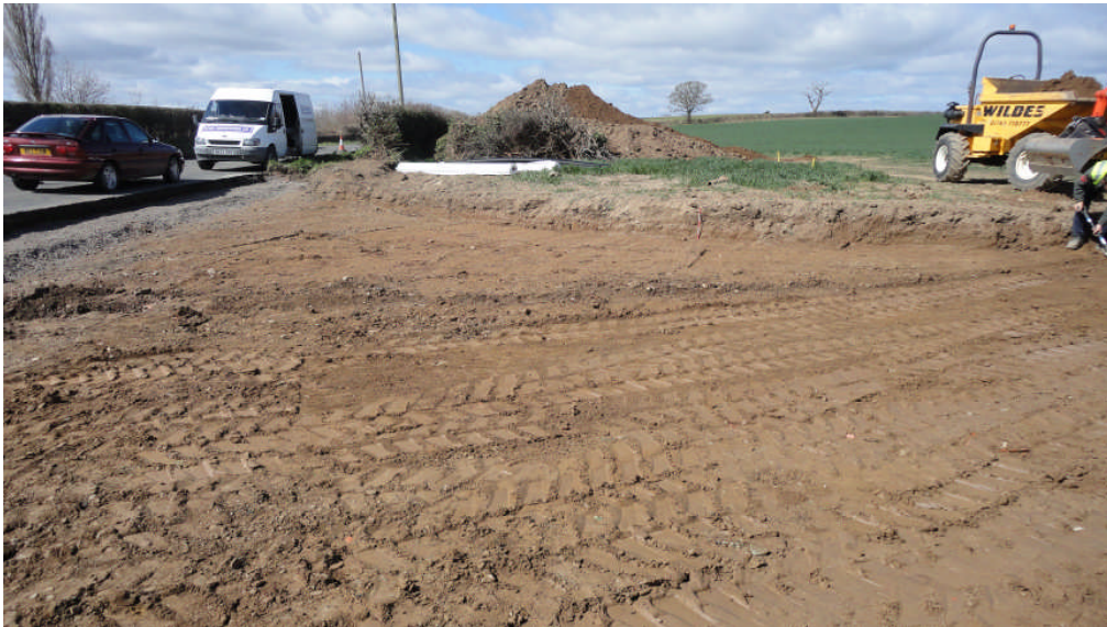
Photo 1: Excavations for the new access on the B4386 road, looking W, scale bar 05m
