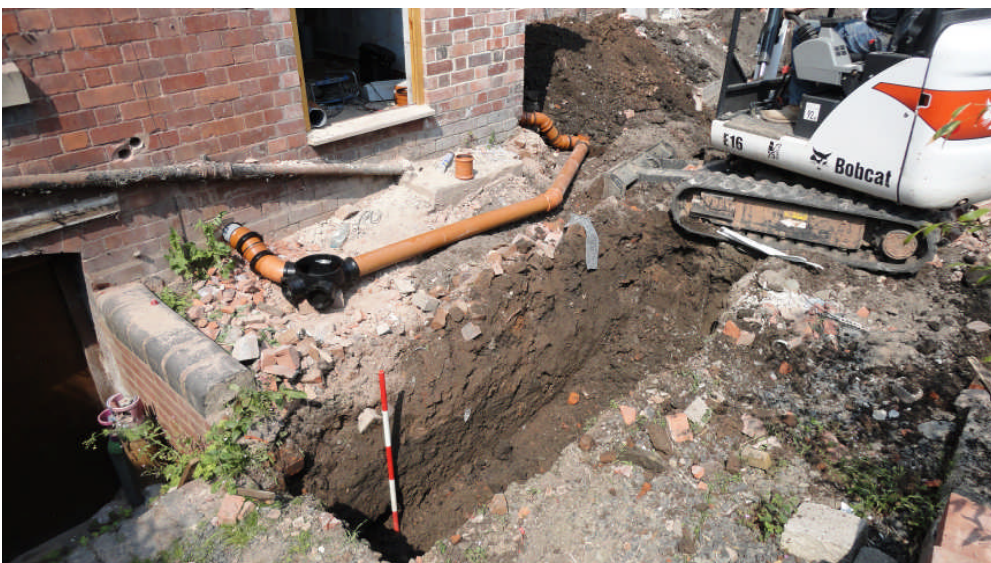
Photo 3: The deposits at the S end of the foundation trench, looking NW, scale 1m
