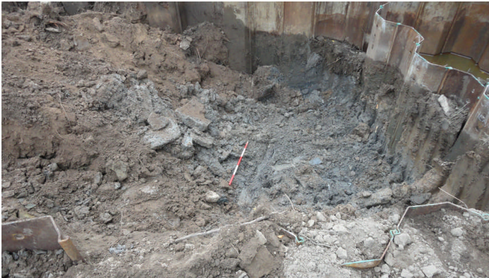
Photo 2: The timber beam and stone bank in the base of the excavations
