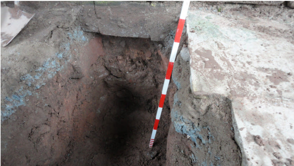
Photo 2: The cobble raft beneath the south aisle wall foundations, looking N (scale bar 1m)
