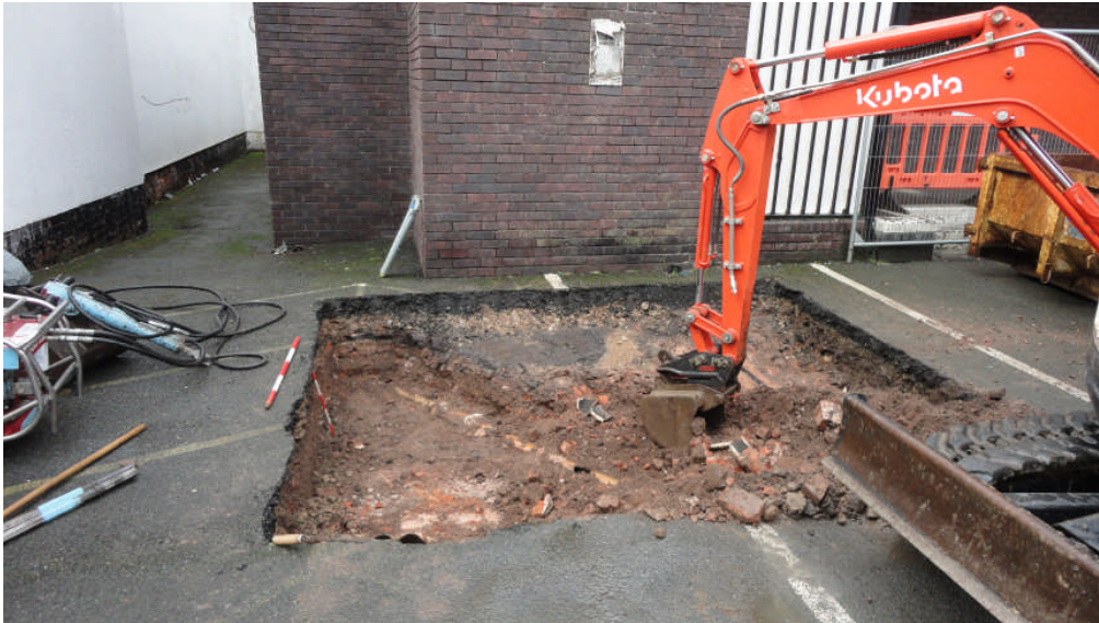
Photo 1: The substation trench at the rear of the site, looking W
