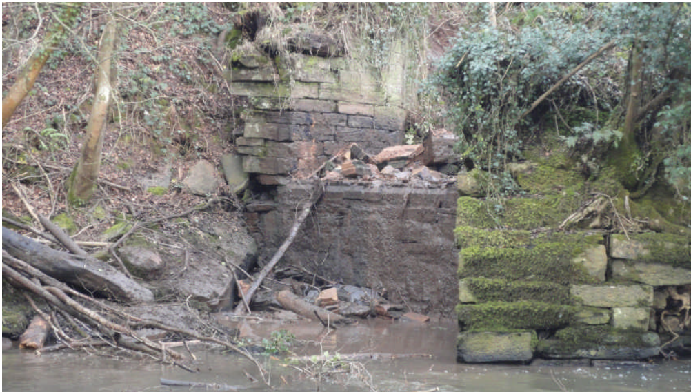
Photo 2: The later courses of the weir at the end of the bypass channel removed
