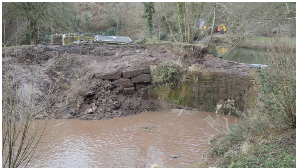
Photo 3: The spoil from the dredged channel used to infill the eroded side of the mill pond.
