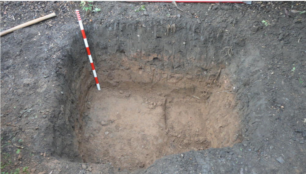
Photo 2: The south-facing section of the foundation pit, looking N; scale bar 1m
