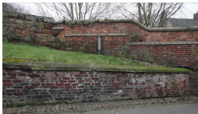
Photo 6: The location of the proposed new opening in the brick section of the outer bailey wall, looking SE
