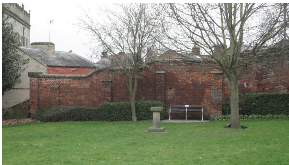
Photo 7: The location of the proposed new opening in the brick section of the outer bailey wall, looking NW
