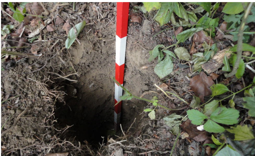
Photo 5: The post hole for the new waymark post, looking SE; scale bar 1m
