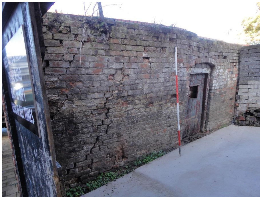
Photo 7: The wall from the rear of 11-12 Mardol, looking NW; scale bar 2m
