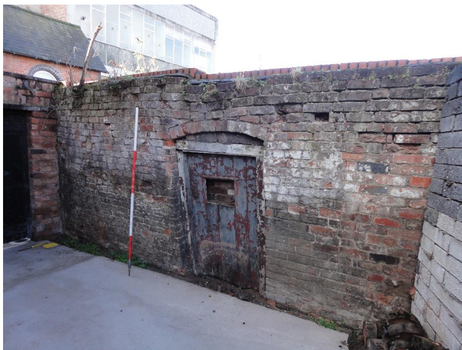
Photo 8: The wall from the rear of 11-12 Mardol, looking SW; scale bar 2m
