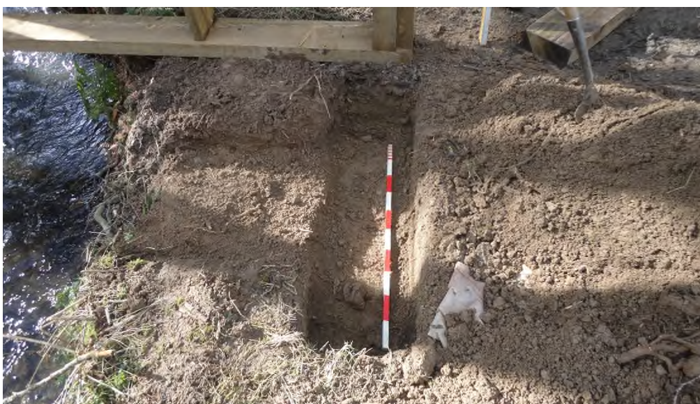
Photo 8: The pit for the north abutment at Lower Mount B, looking W; scale bar 1m
