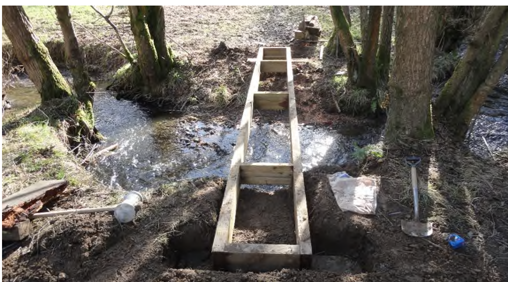
Photo 9: The base for the new footbridge at Lower Mount B, looking S
