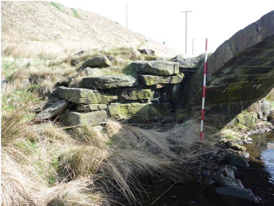
Plate 7: West projection of dry walling to the north access ramp of the bridge, looking northeast
