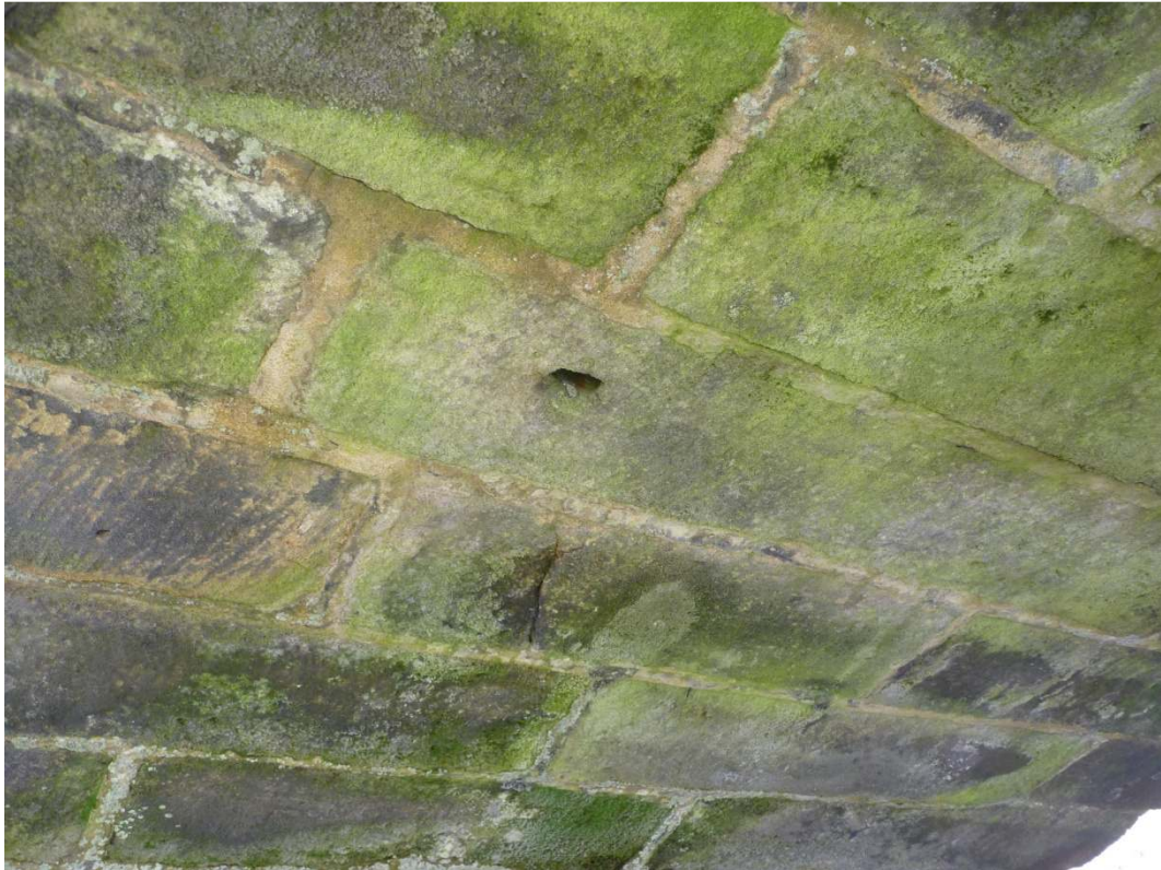
Plate 3: Lewis-type hole to underside of bridge
