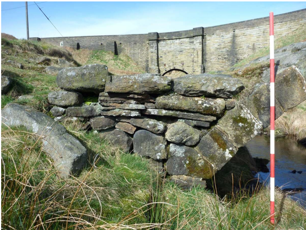
Plate 6: North side of the bridge, showing dry walling to side of access ramp, looking southwest
