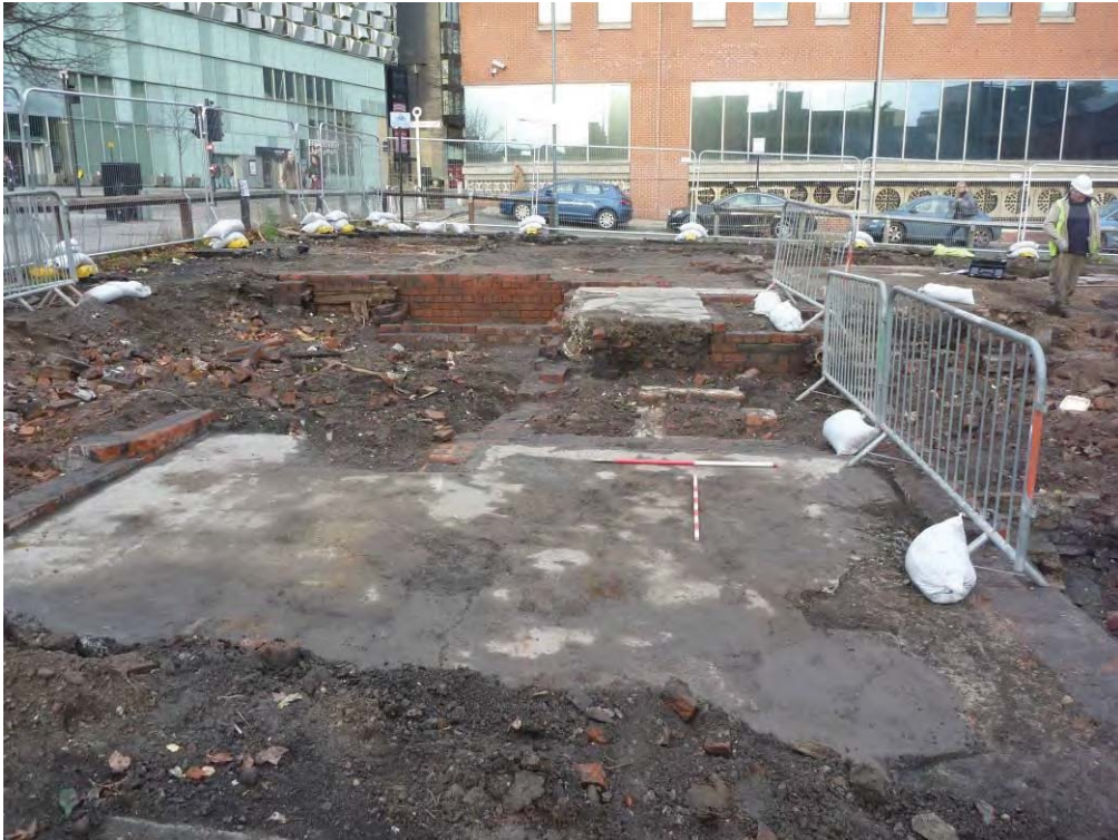
Plate 1: 20 th -century structure on corner of Arundel Gate and Brown Lane viewed from the south-west
