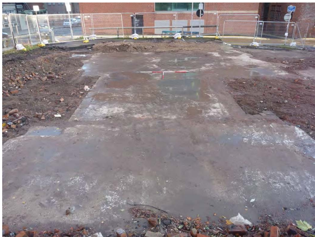
Plate 15: Concrete surface 1067 viewed from the north-west prior to removal during machine strip
