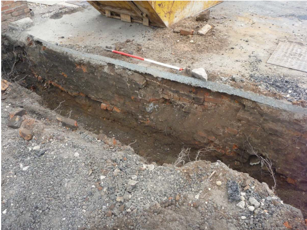
Plate 3: Structure [1005] in north-facing section of south foundation. Viewed facing south-east. 1m scale.
