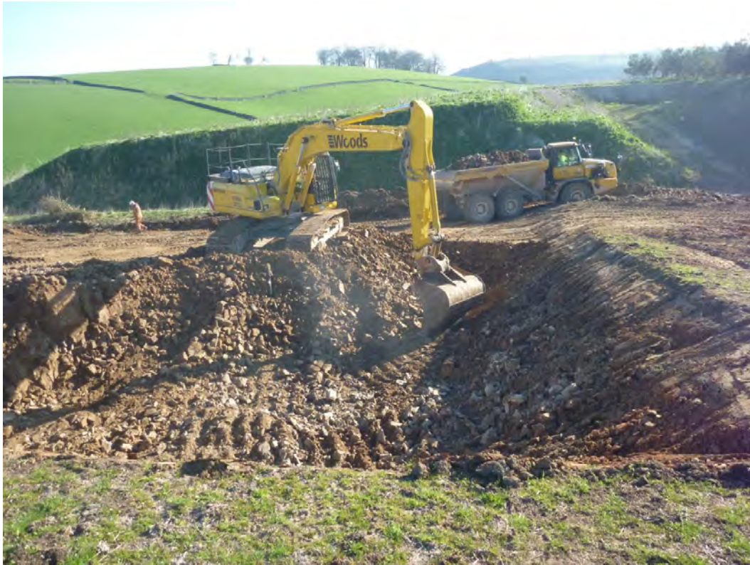
Plate 3: Excavation into the bedrock geology (103) for the footings for the crane pad and Turbine 1. Looking north-east.
