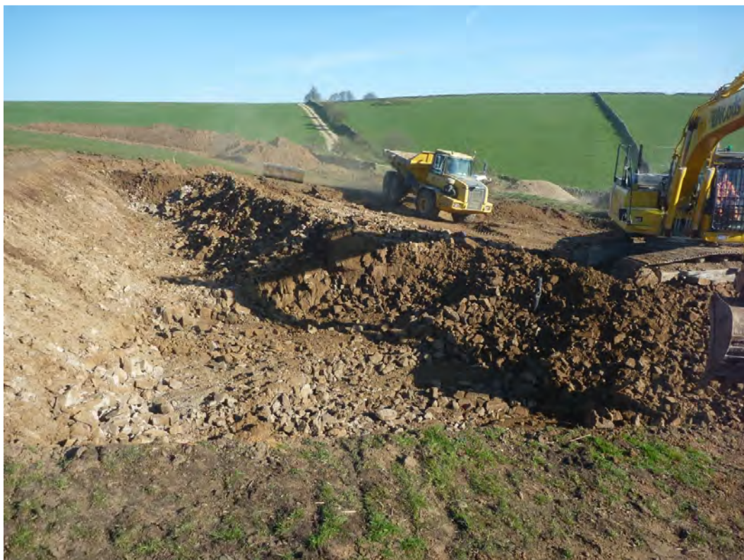
Plate 4: Excavation into the bedrock geology (103) for the footings for the crane pad and Turbine 1. Looking north-west.
