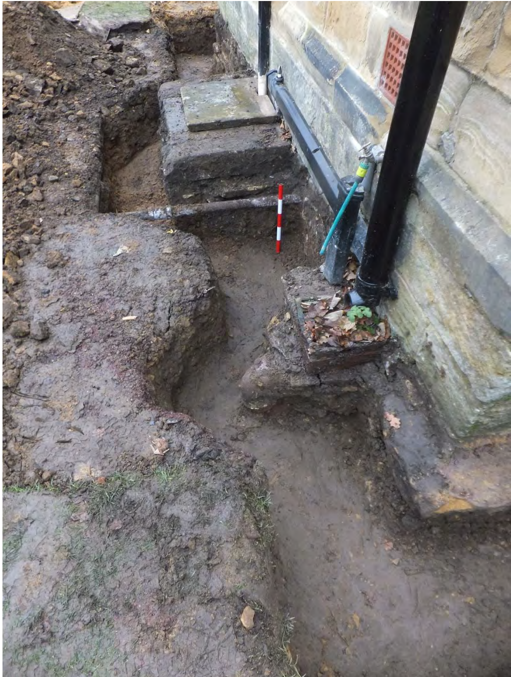
Plate 5: North end of the trench, looking east, showing coal chute (1008). Scale 0.5m.
