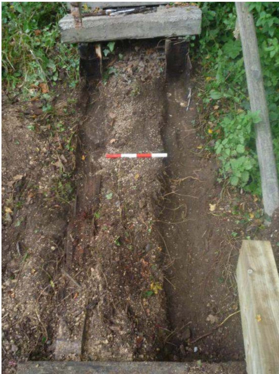
Plate 1: View of site following removal of rotten steps and beams, facing north (scale 0.4m)
