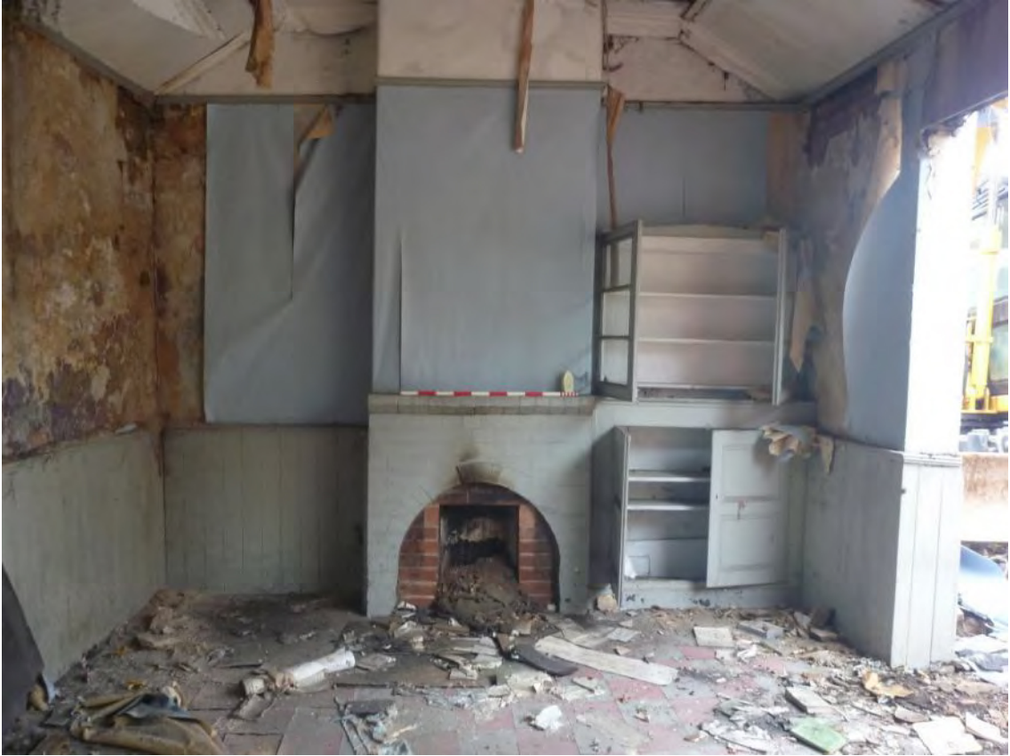
Plate 7: Fireplace and built-in cupboards in the southern half of the building (Room 1). Looking south-west. Scale 1m.
