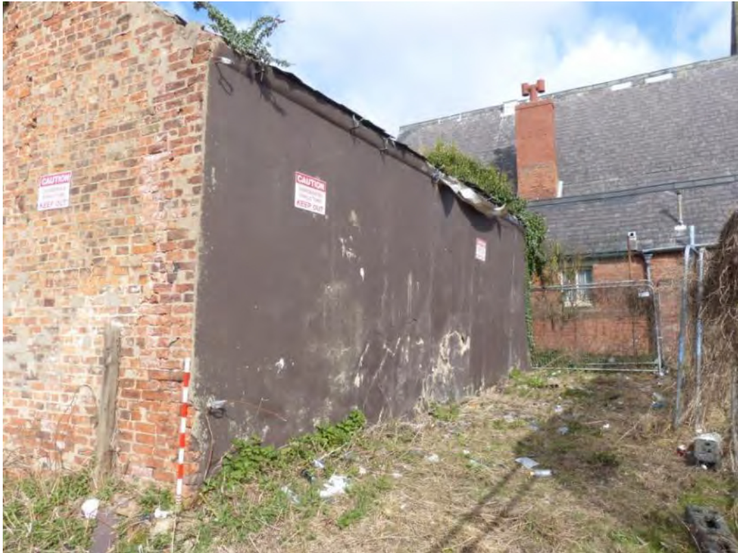
Plate 3: Southern half of the building, showing cement render on the southern elevation. Scale 1m.
