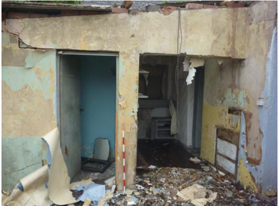
Plate 12: Northern half of the building (Room 2), looking north-east towards a kitchen (left) (Room 3) and toilets (right) (Rooms 4 and 5). Scale 1m.
