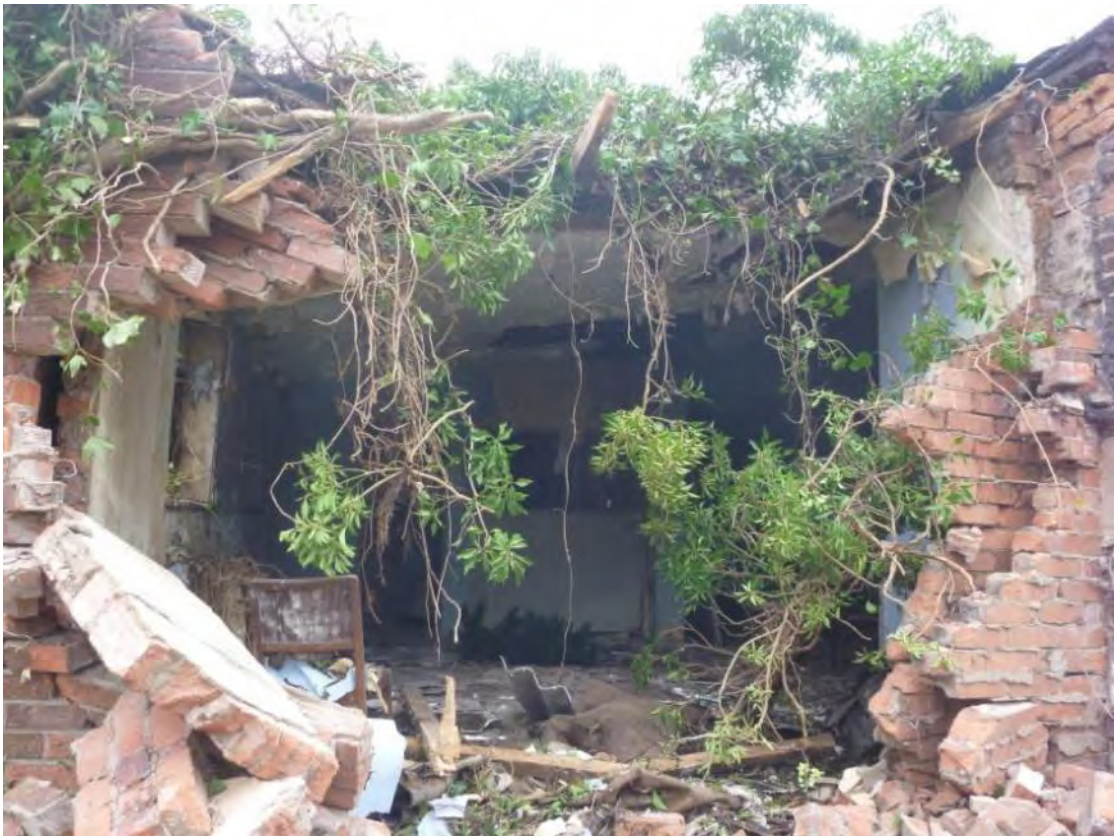
Plate 10: Initial removal of the western exterior wall in the northern half of the building (Room 2). Looking north-east
