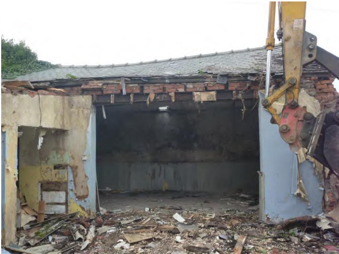
Plate 16: View from Room 2 into the southern half of the building (Room 1). Looking south-east. Scale 1m.
