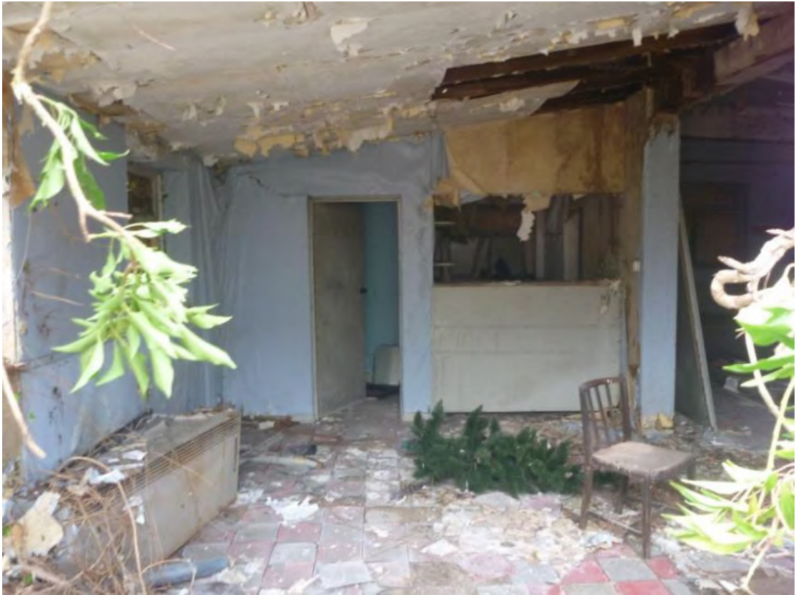
Plate 11: Northern half of the building (Room 2), looking north-east towards a kitchen (left) (Room 3) and toilets (right) (Rooms 4 and 5).
