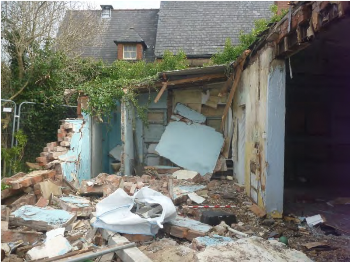
Plate 13: Northern half of the building (Room 2), looking north-east towards a kitchen (left) (Room 3) and toilets (right) (Rooms 4 and 5). Scale 1m.
