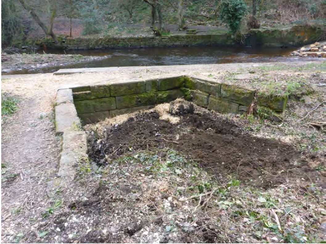
Plate 20: Chamber and bridge (on left) after cleaning modern debris out of the goit
