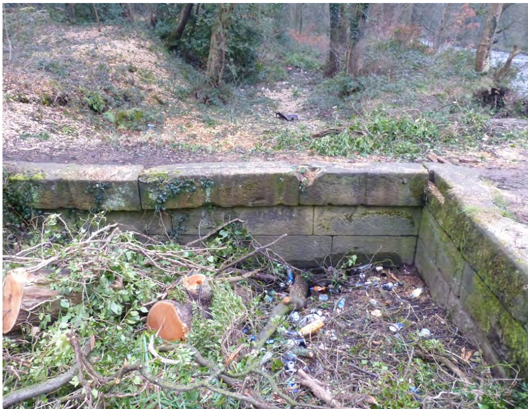
Plate 18: Stone-built chamber looking south across bridge to goit south end (Scale 2m)
