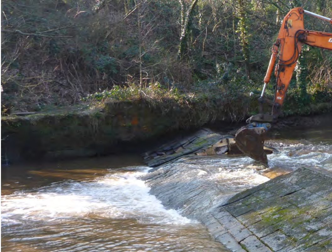
Plate 11: Collapsed section of weir at west end downstream side
