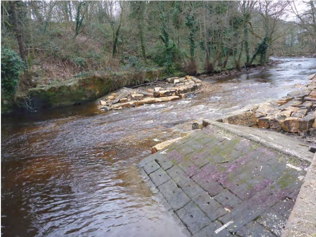
Plate 5: Weir on completion of the works showing both ends of the weir and water flow
