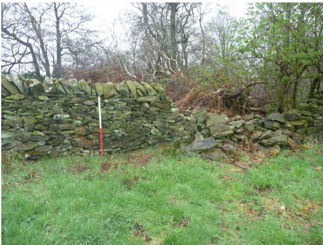
Plate 3: Boundary wall 202 in Rocky Field, damaged by falling tree
