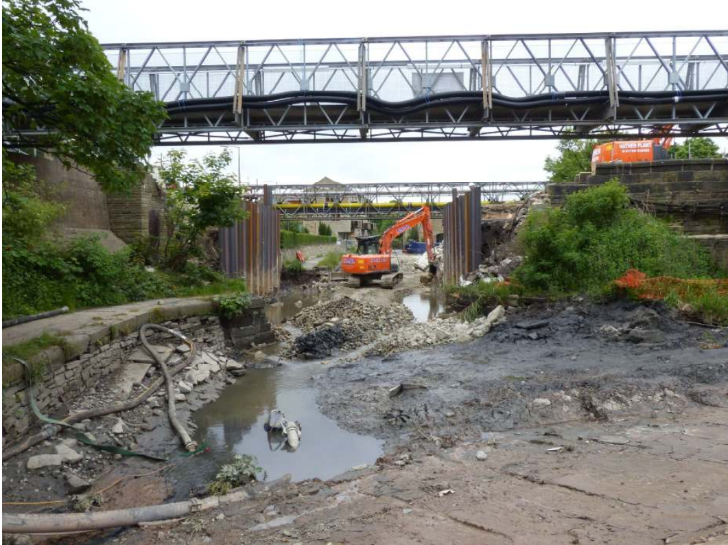
Plate 1: View of the demolished bridge, showing rubble core behind shuttering, viewed facing east
