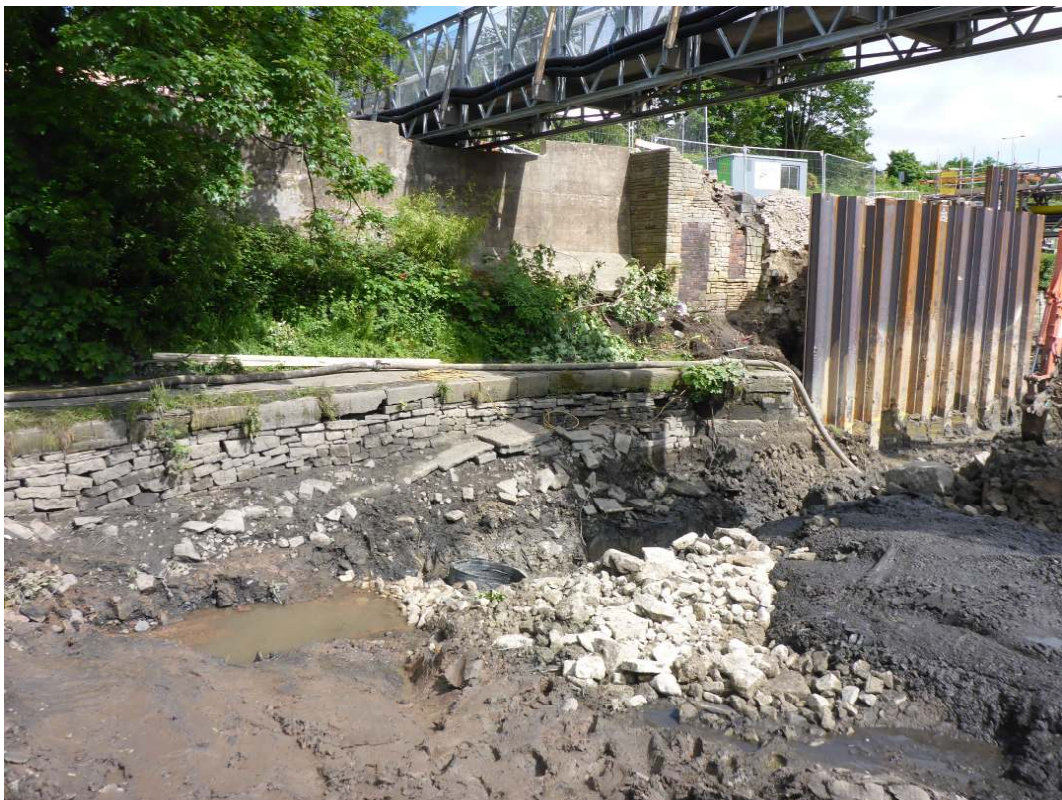
Plate 4: Northern canal wall west of the bridge, with repairs to bridge buttress and possible earlier canal wall, viewed facing north
