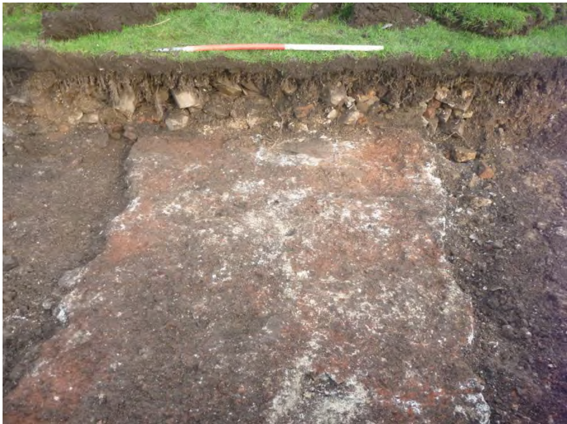
Plate 14: Structure (404), Trench 4, showing the construction cut [405] and demolition backfill (403) in section. Looking north-east, scale 1m.
