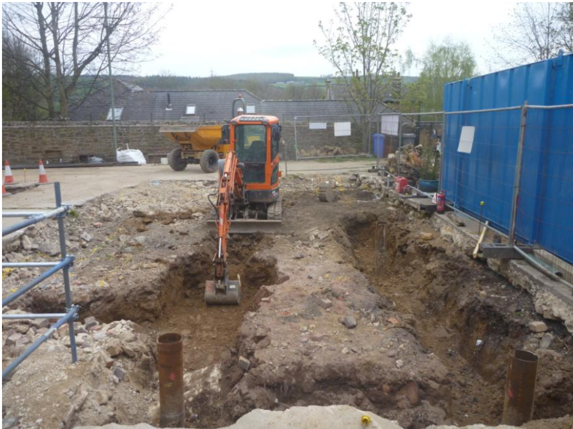
Plate 3: Working shot of the excavation of the footings within Area A. Looking east, scale 0.4m
