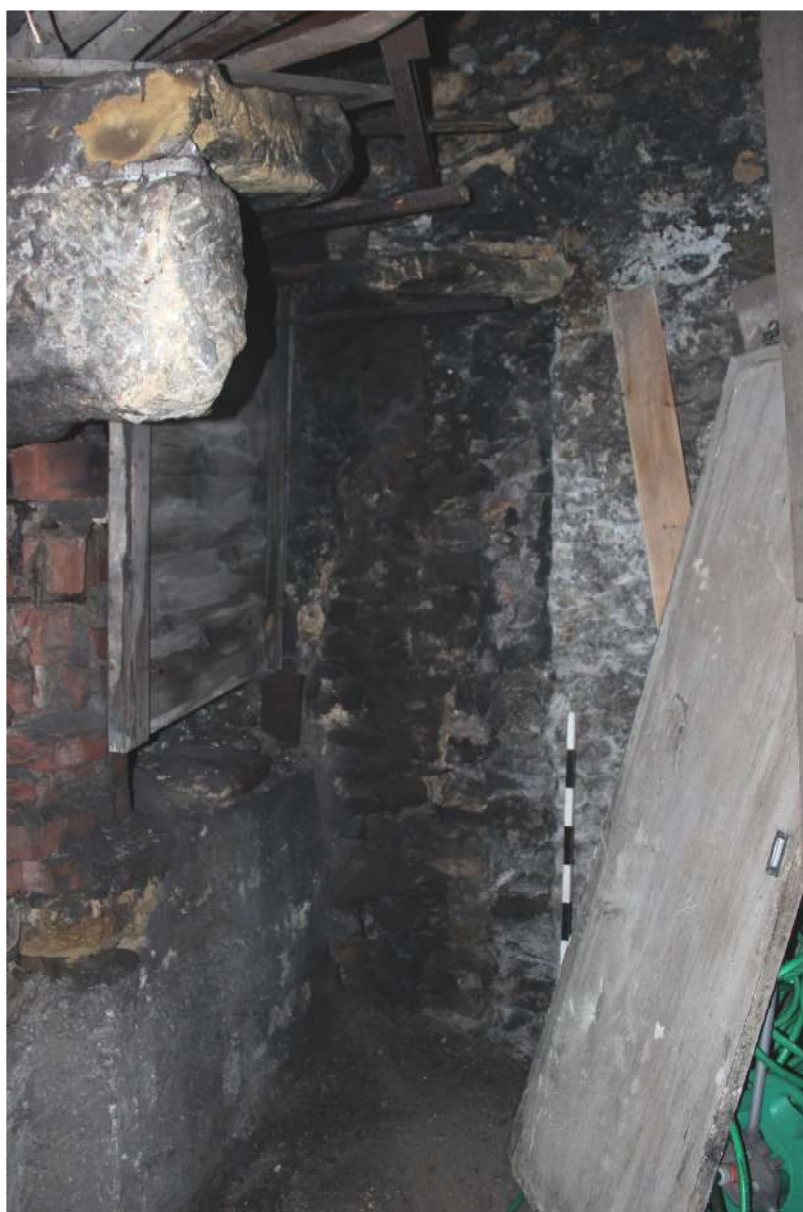
Plate 16: Dark stain on wall indicating the original extent of the hearth
