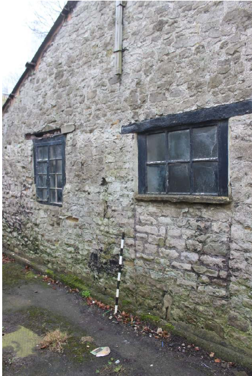
Plate 7: Enlarged window to left and, to right, a partly infilled former doorway in the east elevation
