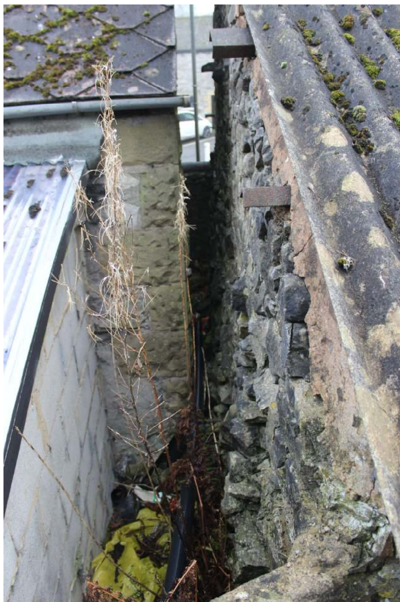
Plate 10: Roughly faced walling on the west side, with a narrow gap to the neighbouring property
