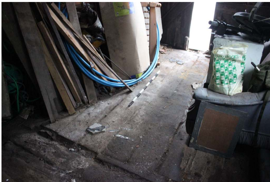
Plate 18: Sloping wooden flooring between the street entrance and the middle of the smithy
